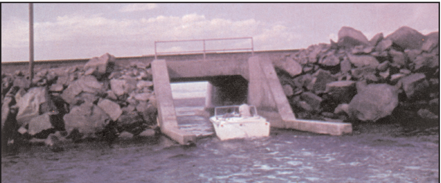
One of the two 15-foot-wide by 20-foot-deep culverts in the rock-fill portion of the causeway. Photo taken during low lake level (1960-1962).
