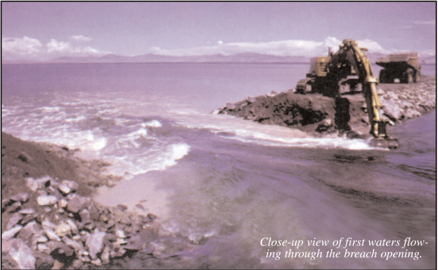
Breach in the SPTC causeway, near Lakeside, looking north-east. Photo by P.A. Sturm.
