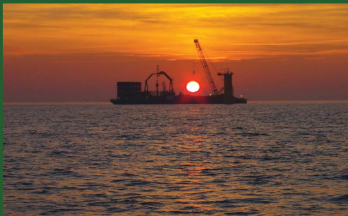
A cable installation barge at sunset during the construction of the Lynn Offshore Wind Farm
