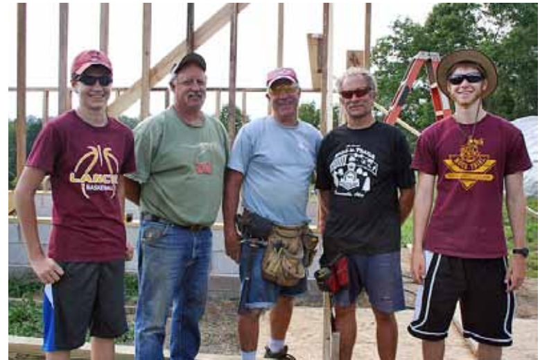
Team Guindon builds the chicken house. Left to right: Matthew Hammer, Don Guindon '74, Dale Guindon '67, Leonard Guindon '70, Rob Hammer. Matthew and Rob are the children of Janet Guindon Hammer '76.
