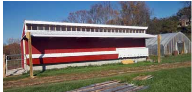
The new chicken house is home to 100 hens, who will provide fresh eggs daily to meet all the school's needs. The project was funded by donations in memory of former farm manager Cliff Guindon '41.
