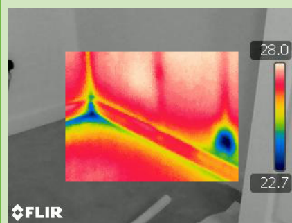
Figure 12: Cold spot on external wall
