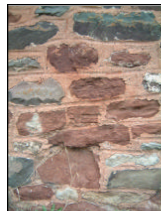
The two local sandstone types. The softer red, needs an equally soft lime-based mortar to avoid more rapid deterioration.
