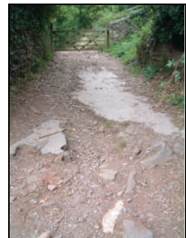
Damage to footpath surface due to water erosion
