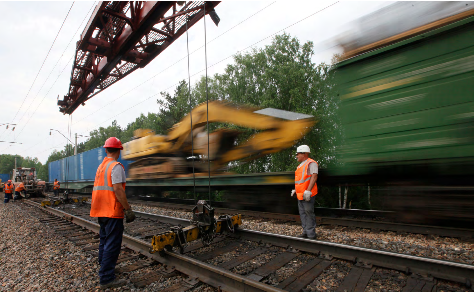
LINE MANAGEMENT: Workers replace track in the Taiga district of the Trans-Siberian Railway, which some envisage as an alternative route for transporting goods from China to Europe. REUTERS/ILYA NAYMUSHIN
