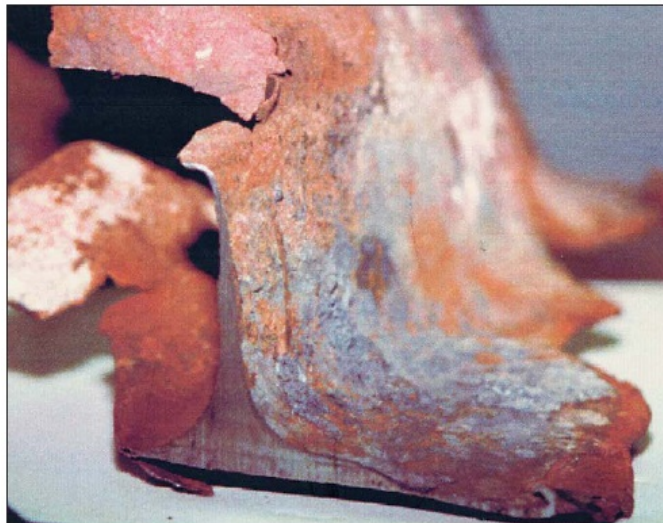
Figure C-2 Closeup view of eroded wide-flange beam section.
