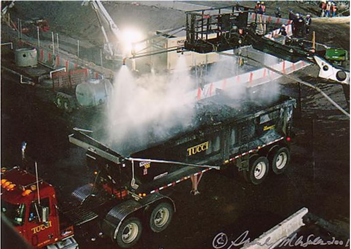
Dust suppression was critical considering the asbestos and lead, etc., in very fine particles (photo unknown source)
