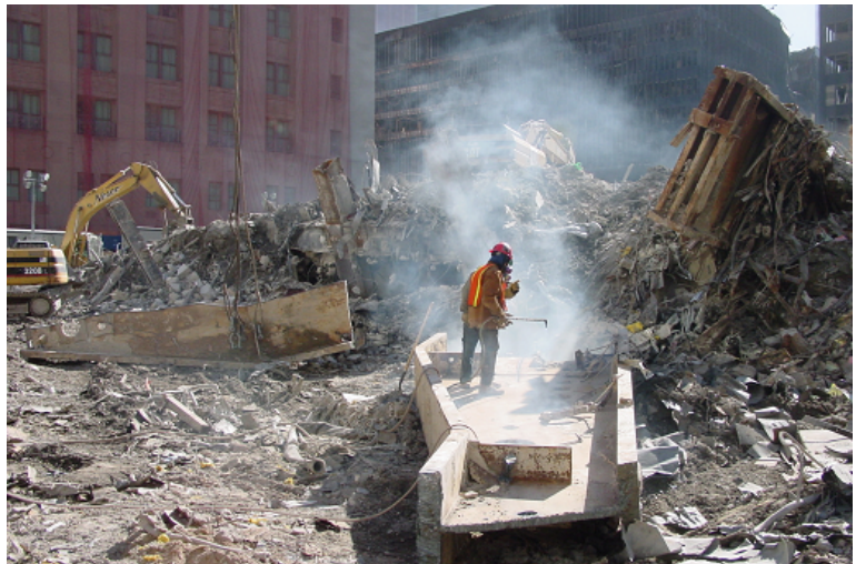
WTC 7 debris pile Oct. 18. Source: NIST [ enlarge photo ]
