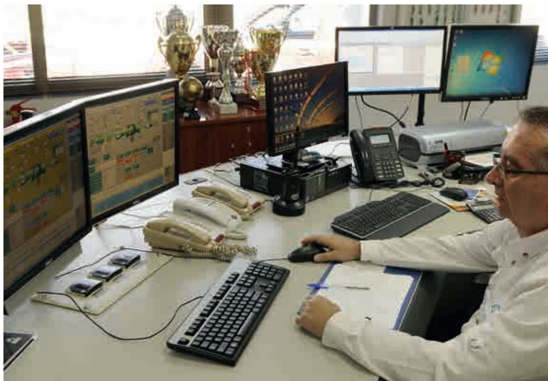
Candelaria Power Plant
