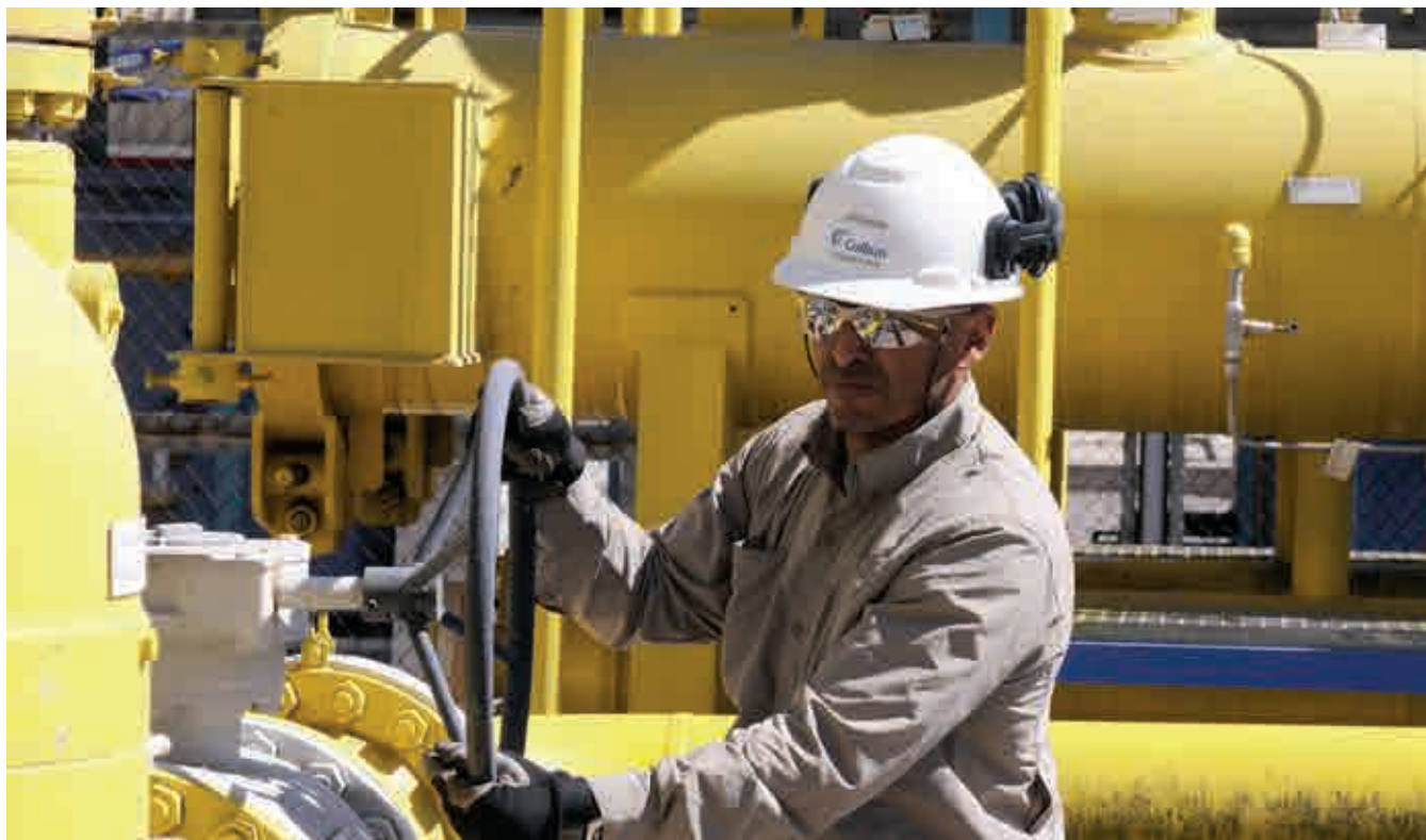
Santa María Power Plant
