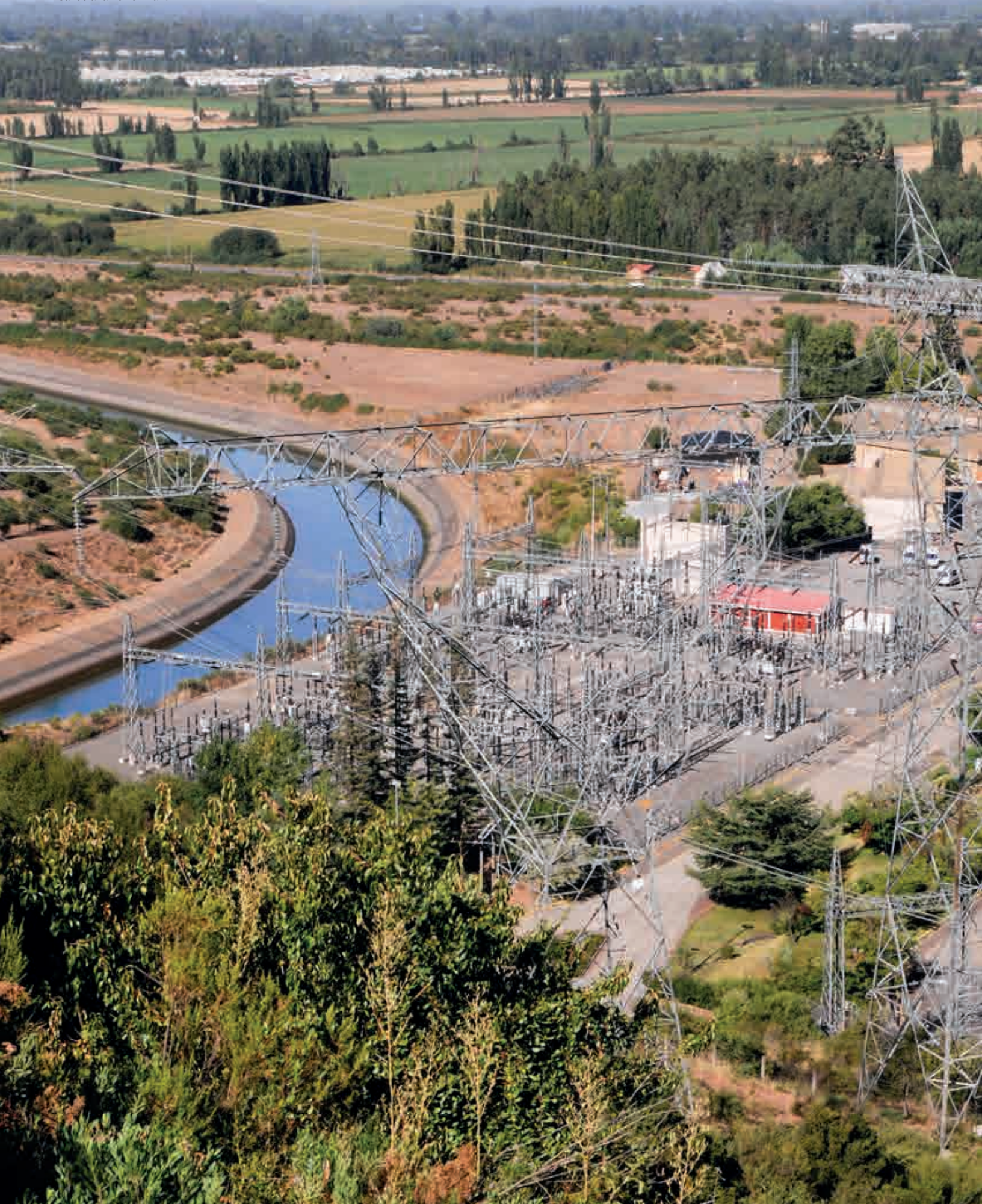
Candelaria Power Plant
