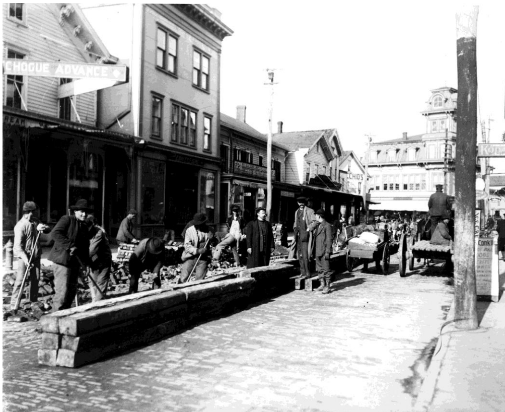
Trolley Line construction team works on S. Main St. extension line, Patchogue, NY, on November 13, 1907 (Photo by Howard S. Conklin, Courtesy Long Island Advance)
