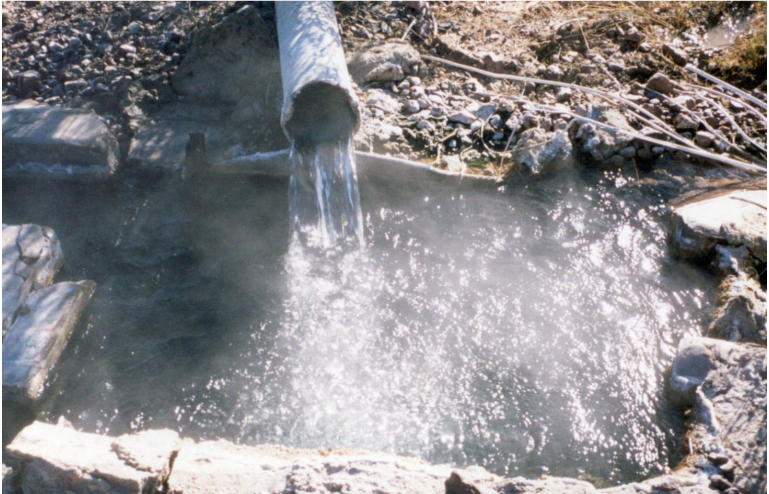
Figure 2.2: Bore outlet pipe and pool of the New Lorne Bore
