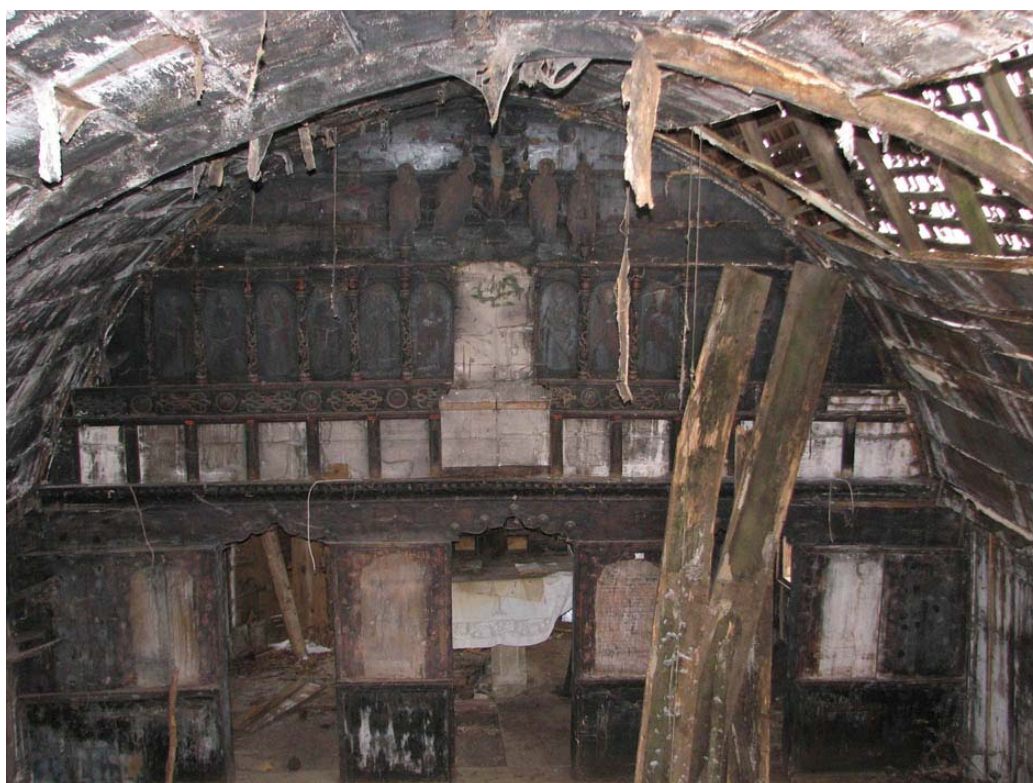
Figure 8 – Vault in collapses
