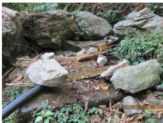
Collection chamber working with makeshift repairs in Thachambu W.S.P. in Thachambu VDC of Taplejung
