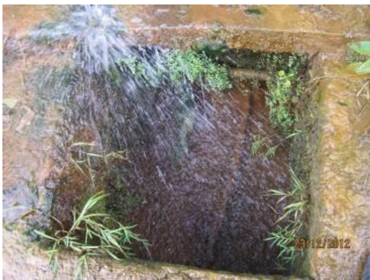
Leaking pipe in Chhatyungaira W.S.P.in Ghyalchock VDC of Gorkha
