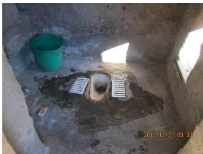
Toilet in Rupertola W.S.P in Dhamana VDC of Bajhang
