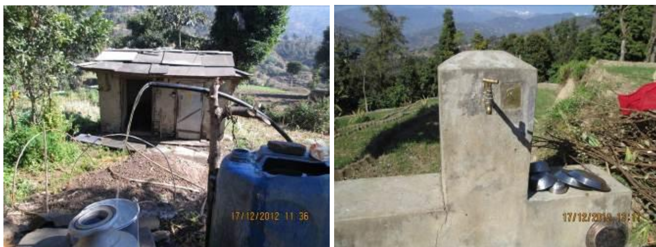
A cut pipe tap stand and properly functional tap stand in Dhije Mul W.SP. in Shikarpur VDC of Sindhupalchowk district
