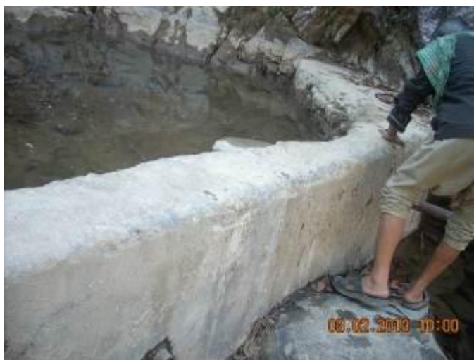
Intake of the Dhungra Khola W.S.P. in Shikharpur VDC of Makwanpur
