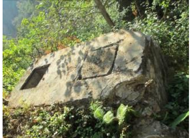
Cracking collection chamber in Nakedanda W.S.P in Jaidi VDC of Baglung
