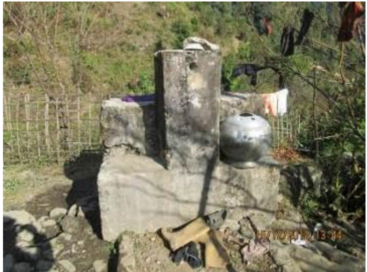
Non-functional tap stand in Change Khola W.S.P. in Yamphudin VDC of Taplejung
