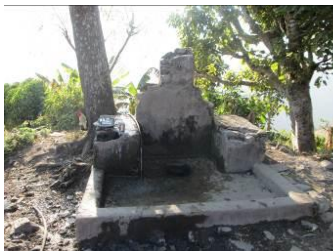
A broken tap stand with water still supplied by a loose pipe in Khulikhola W.S.P. in Burtibang VDC of Baglung district
