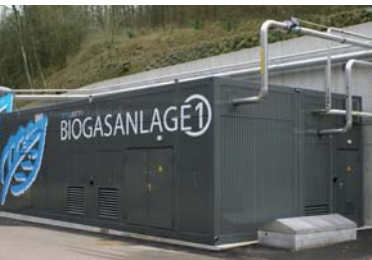
The raw gas for the upgrading plant in Bern (Switzerland) is yielded from sewage gas and waste.
