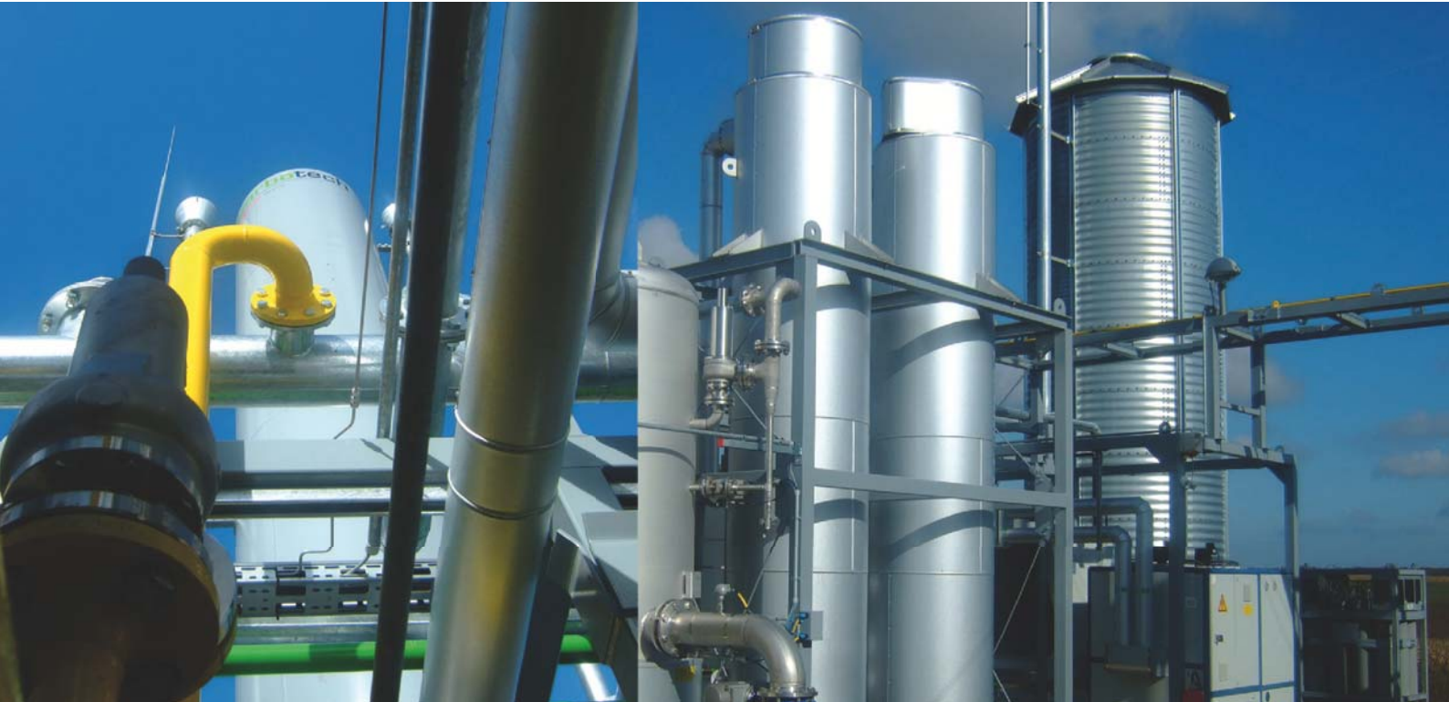
Biogas upgrading plant Emmertsbühl/Blaufelden
