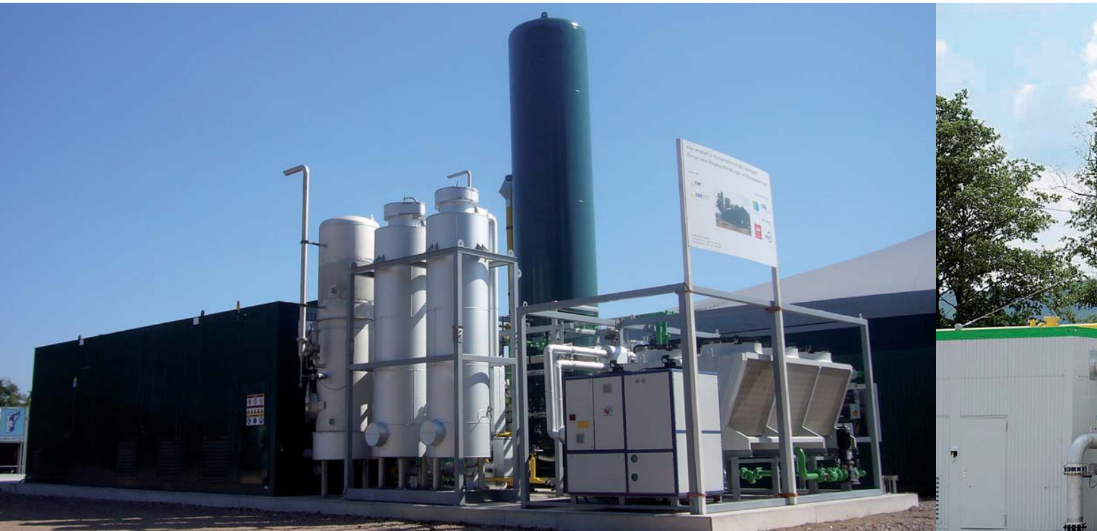
Biogas upgrading plant, Wüstring/ Oldenburg, Ostfriesland
