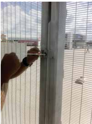
It is preferable to unlock all exits and replace the lock with cable ties, as these can easily be overcome by a crowd wishing to exit in an emergency.
