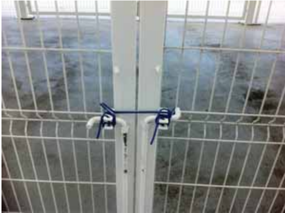
Gates must be opened and manned once spectators are inside the stadium. Failure to open gates during mass evacuation leads to loss of life.
