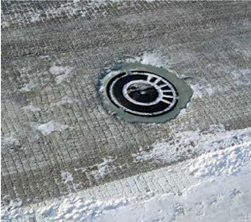
Spray head in bridge deck
