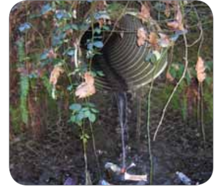
Untreated runoff and trash
