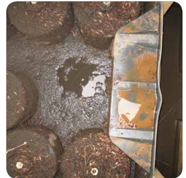
A sediment-filled stormwater vault
