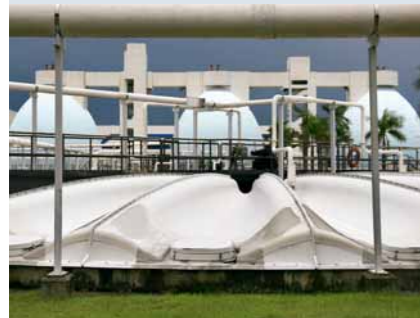
The Kranji NEWater treatment plant transforms wastewater into potable water.
