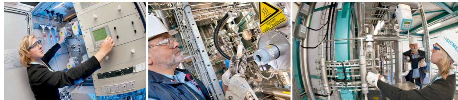
To ensure optimal operation, technicians must continually measure parameters such as the CO 2 and SO 2 content of flue gas (left, center), as well as flue gas volume flows (right).
