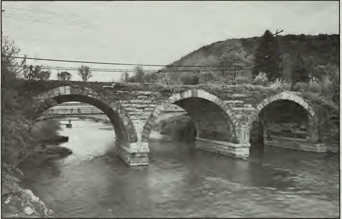
Photo 42. View of south side of Standing Stone Creek Bridge. Photo by Jet Lowe.
