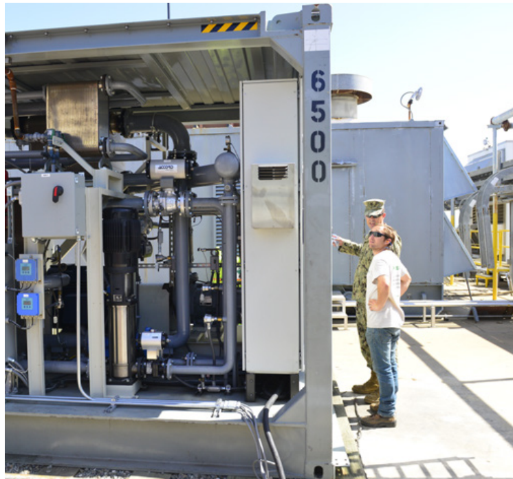
Two men monitor the start-up of a new Electrathem Organic Rankine Cycle, the base main power plant. The unit is an alternative, or Green, energy system that takes heat from different systems and converts it into usable energy or electricity.
