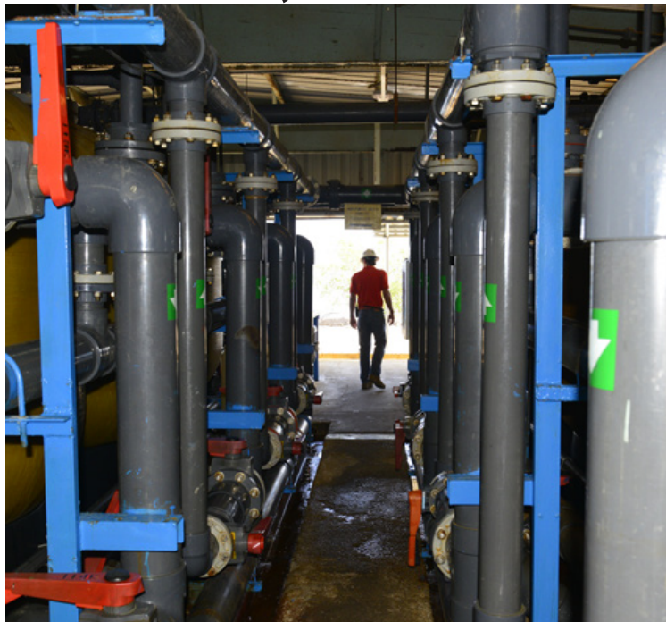
Steven Vickery, utility management branch head at Naval Facilities Engineering Command, conducts a routine walk-through of the water purification plant at the Desal Plant, Guantanamo Bay, Cuba.
