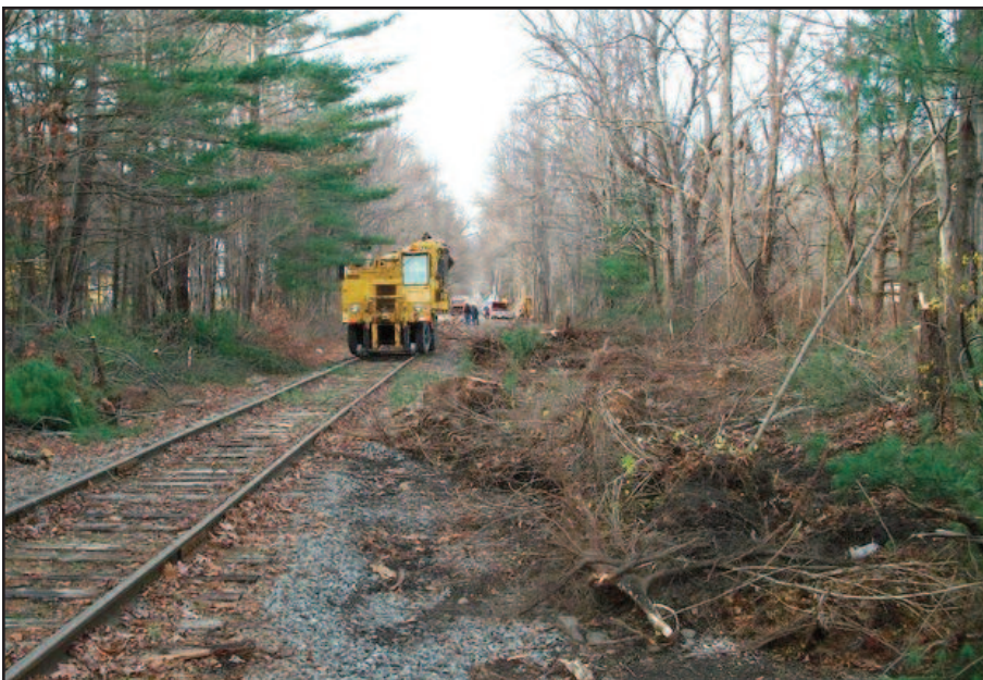
Preliminary work for a new storage siding at MP 24.75 was under way on November 19, 2011. Construction of this siding will increase storage capacity on the railroad, and allow us to park work equipment without blocking the main line. Photo by Ernest Hunt
