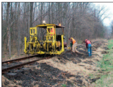
On April 16, volunteers were spiking ties at MP 25.6, part of our planned routine maintenance of the line.
