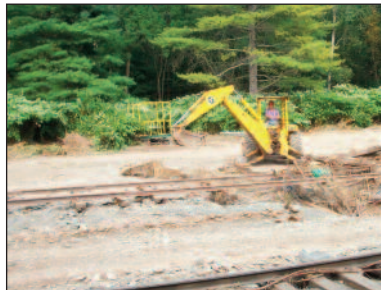
CMRR President Earl Pardini removes debris from the equipment siding in Phoenicia with a small backhoe on September 3.
