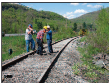
The CMRR track crew tamped and leveled the track at Campground Curve at MP 26.5 on May 7.
