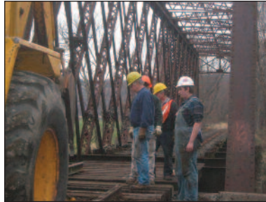
The C9 Bridge Crew at work, putting back rail on the bridge over the Esopus on November 13. Photo by Ray Farrell
