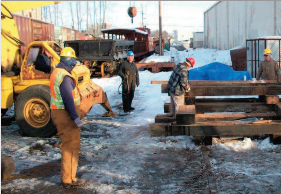
Our big winter project was notching new timbers for Bridge C9. About 300 are needed to complete the repair. Earl Pardini is using a chainsaw to notch these timbers on February 19.
