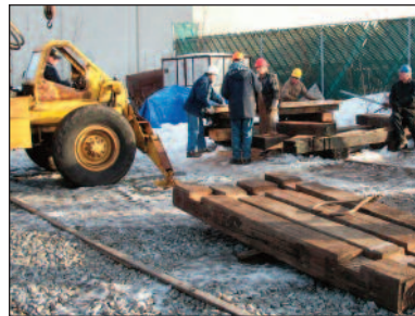
Four completed bridge timbers are in the foreground on February 19. The work was performed at our Cornell Street Yard facility.
