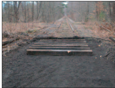
The first seven ties were installed at MP 24.75 for the new storage siding at Longyear Switch on December 31. Photo by Ernest Hunt
