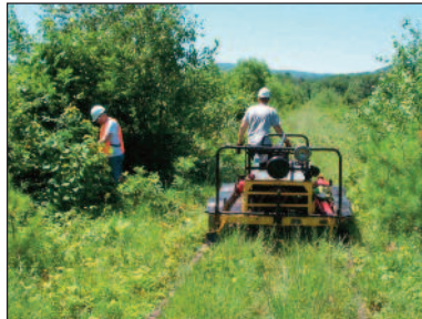
On July 9, volunteer brush crews were out cutting trees over 1 inch in diameter in preparation for running the sickle bar cutter out beyond the rails to improve clearances and reduce encroachment.
