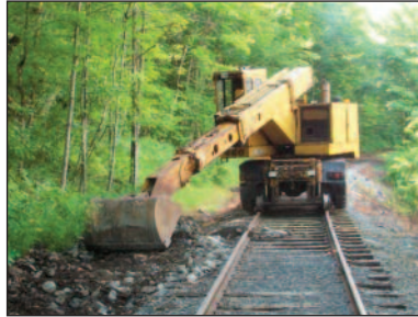
On July 31, we used our hi-rail Gradall to spreading stone at MP 23.3.
