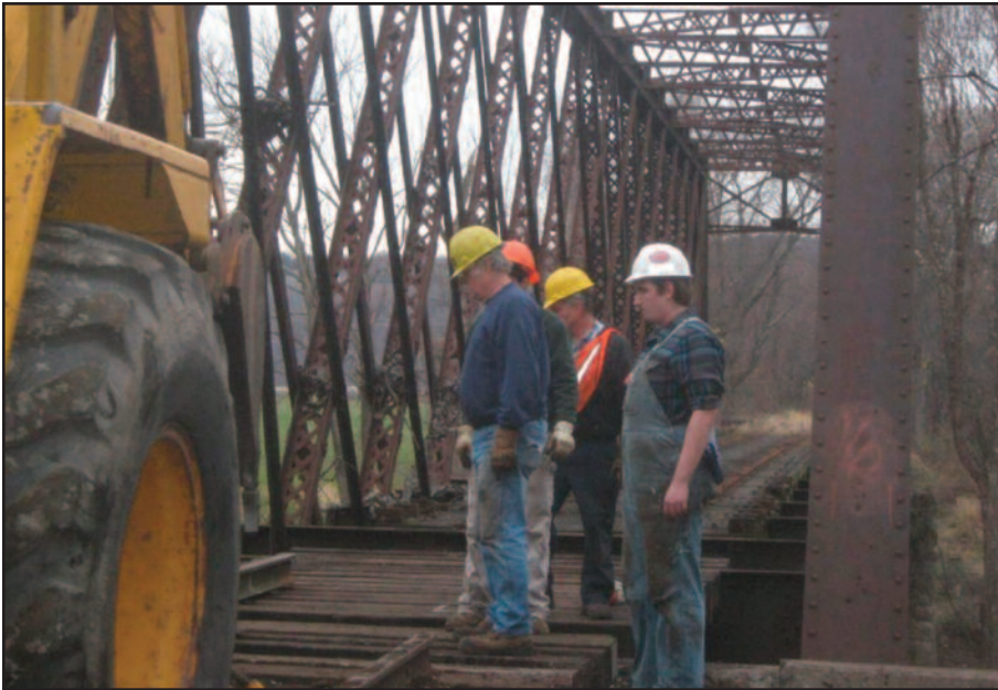
Volunteer crews continued re-decking Bridge C9 in Kingston through the end of 2011. Completing the repair and recertification of this span will allow us to further expand the train ride towards Ashokan Reservoir from Kingston. Photo by Ernest Hunt
