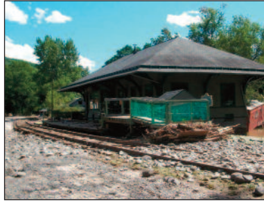
The yard and tracks were flooded, and the entire area suffered from scouring when the Esopus rose and chose the railbed as the path of least resistance. Photographed on August 29.
