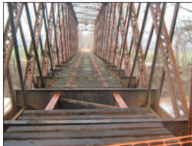
The first of new timbers were placed on Bridge C9 by the end of the year. Photo by Ernest Hunt
