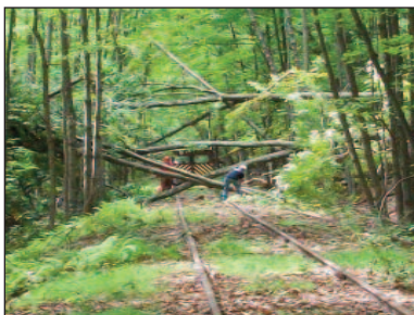
The brush crew removed many trees downed by Hurricane Irene, seen here at MP 14.2.
