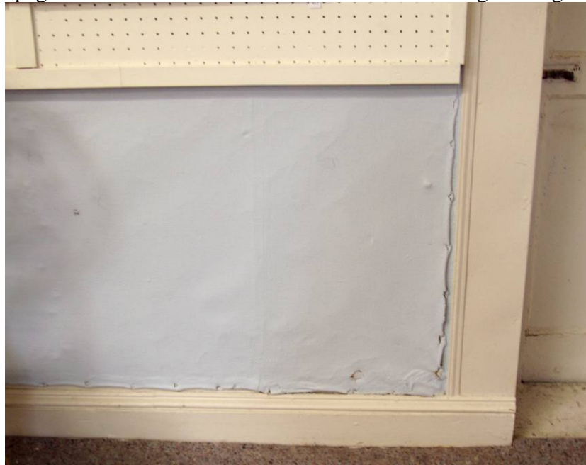
Figure B92. Second floor studio, lower portion at the eastern wall at the south, showing early monks' cloth under the layers of paint.
