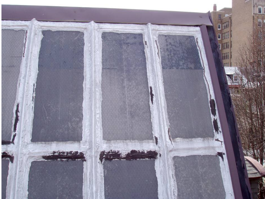
Figure B101. Skylight exterior, western corner. Note the variety of materials surrounding the window panes.
