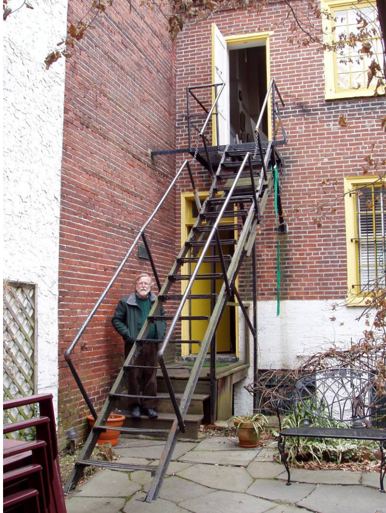
Figure B13. Rear façade, southern end showing the iron fire escape. (Michael Guinn included in the photograph.)
