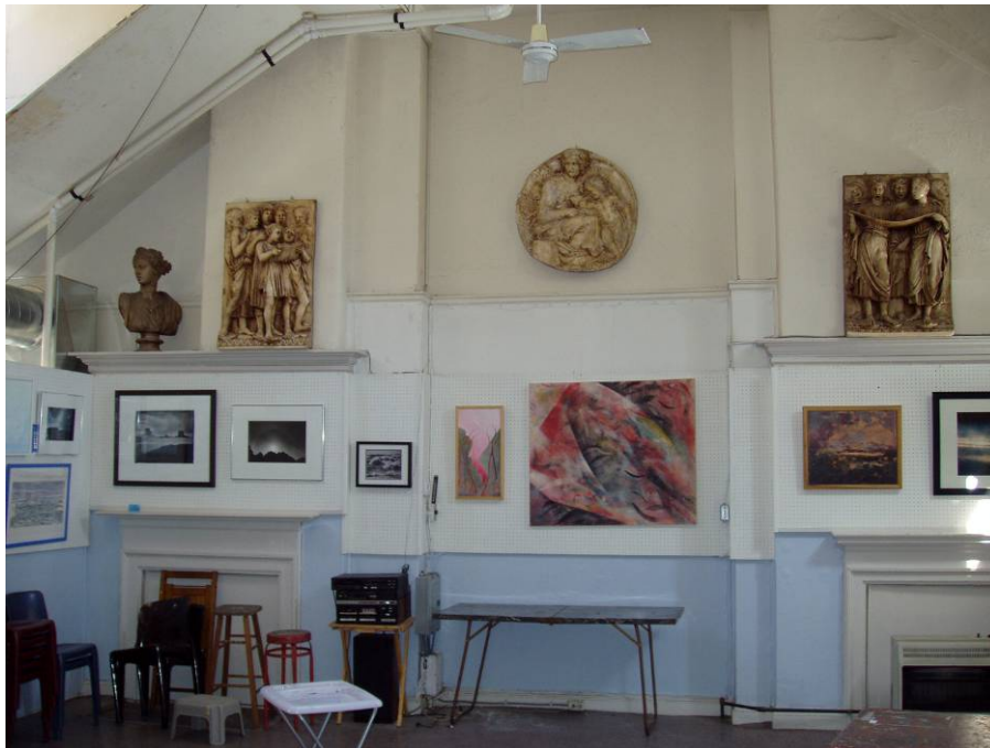
Figure B83. Second floor studio, northwest corner. Note the original fireplaces boarded up.
