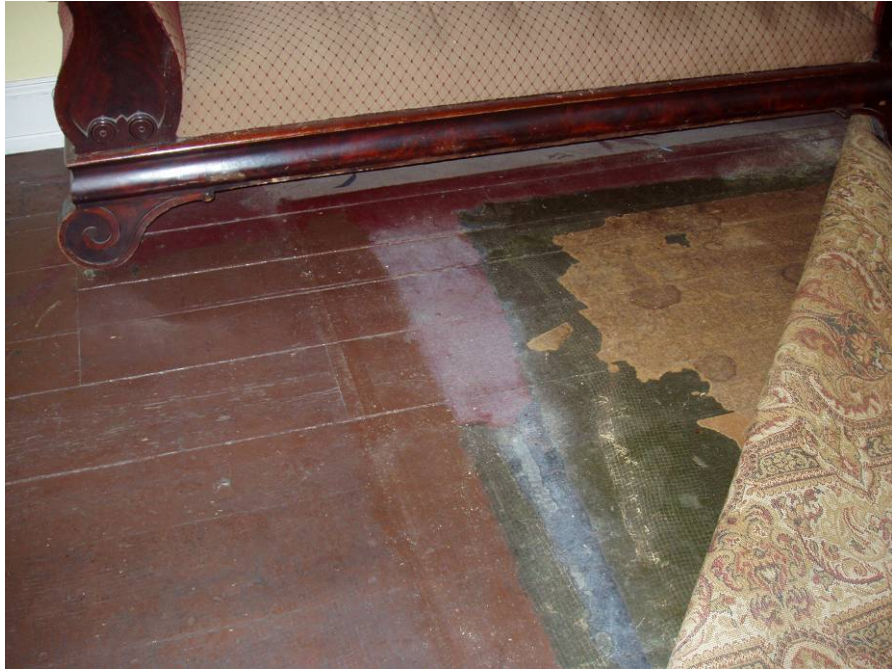
Figure B51. First floor main room, original floors with paint and matting residue.
