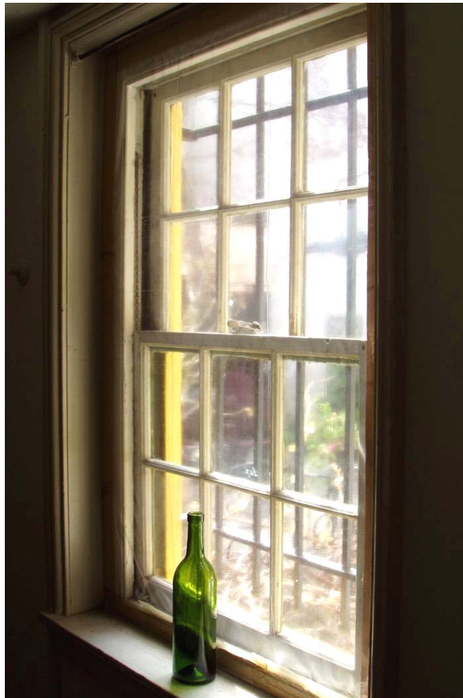
Figure B57. Window in the first floor rear stairwell extension, south wall.
