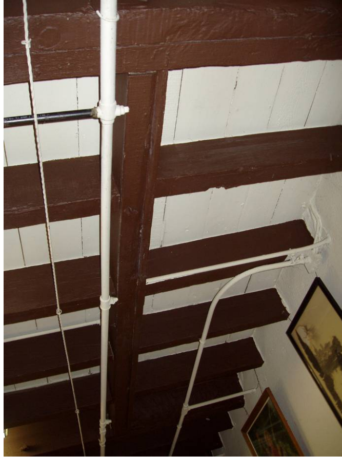
Figure B35. Basement main room, ceiling with water pipes and electrical wires. Note the framed opening where the original stairs were located.
