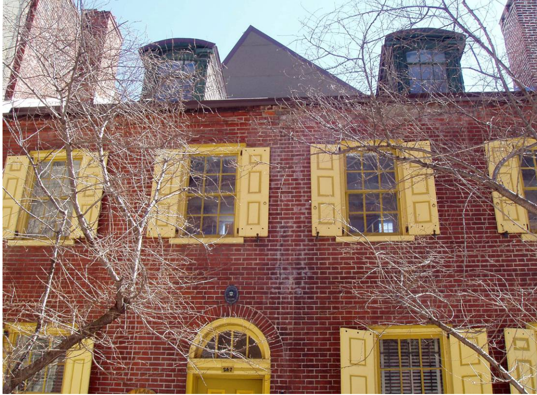
Figure B8. Exterior façade of 247 S. Camac Street, second story. Note the efflorescence on the brick between the middle windows.
