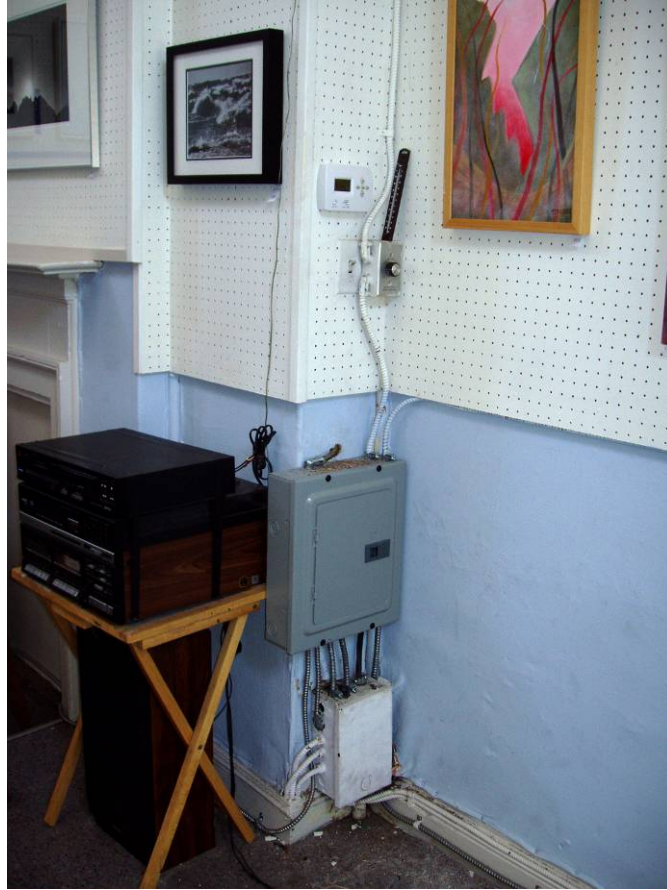
Figure B98. Second floor studio, electrical control panel and newly installed thermostat on the north wall.
