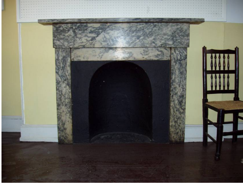
Figure B53. First floor main room, northwest corner. Matching King of Prussia marble mantle, but the stove has been removed and the interior filled.
