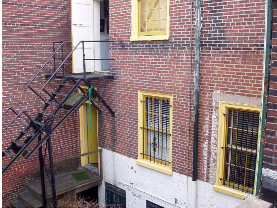
Figure B12. Rear façade, southern half. Note the rust stains on the brick below the fire escape and the peeling paint on the lower part of the wall.
