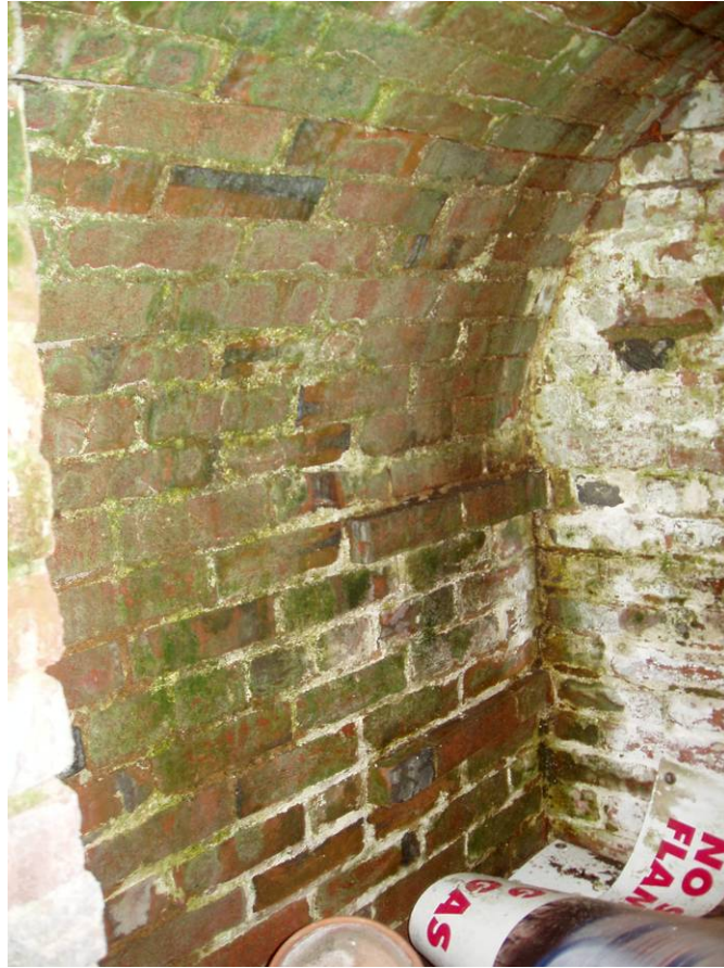
Figure B23. Rear garden retaining wall, northern vaulted storage area. Note the shelf brackets along the wall.
