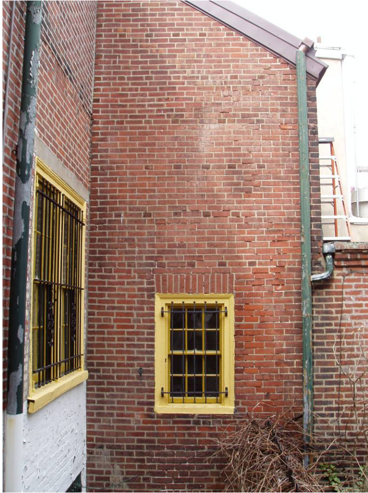
Figure B15. Rear façade, southern face of the rear stairwell extension on the north end. Note the areas of mortar loss on the wall.
