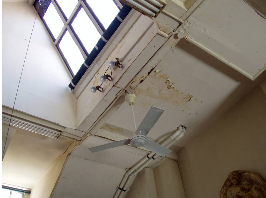
Figure B87. Second floor studio skylight, north section. Note the severe water damage in the ceiling from the leak in the skylight, also the HVAC pipes coming into the room from the ceiling.
