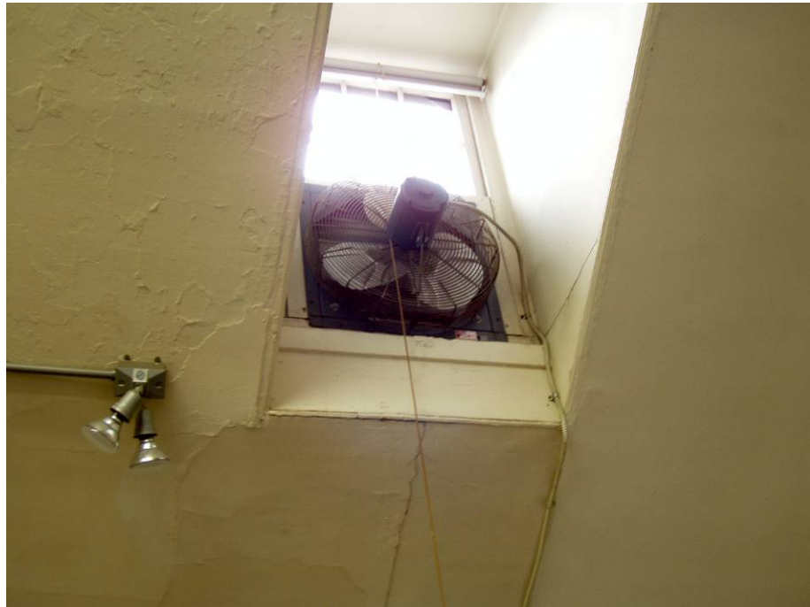
Figure B94. Second floor studio rear southern dormer window. Note the cracking and flaking in the wall plaster around the window.
