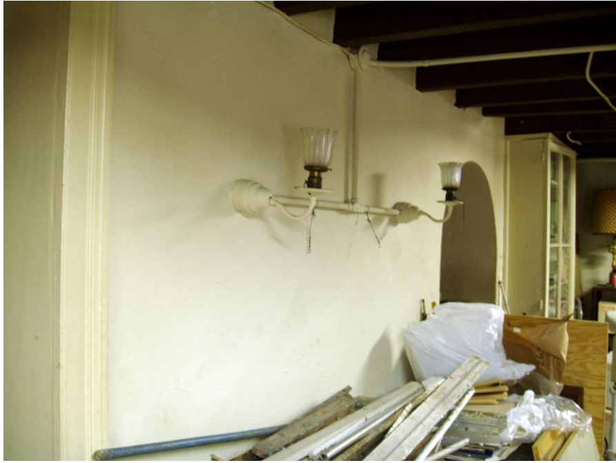
Figure B34. Basement main room, south wall. Note the original gas wall fixtures, updated for electricity.
