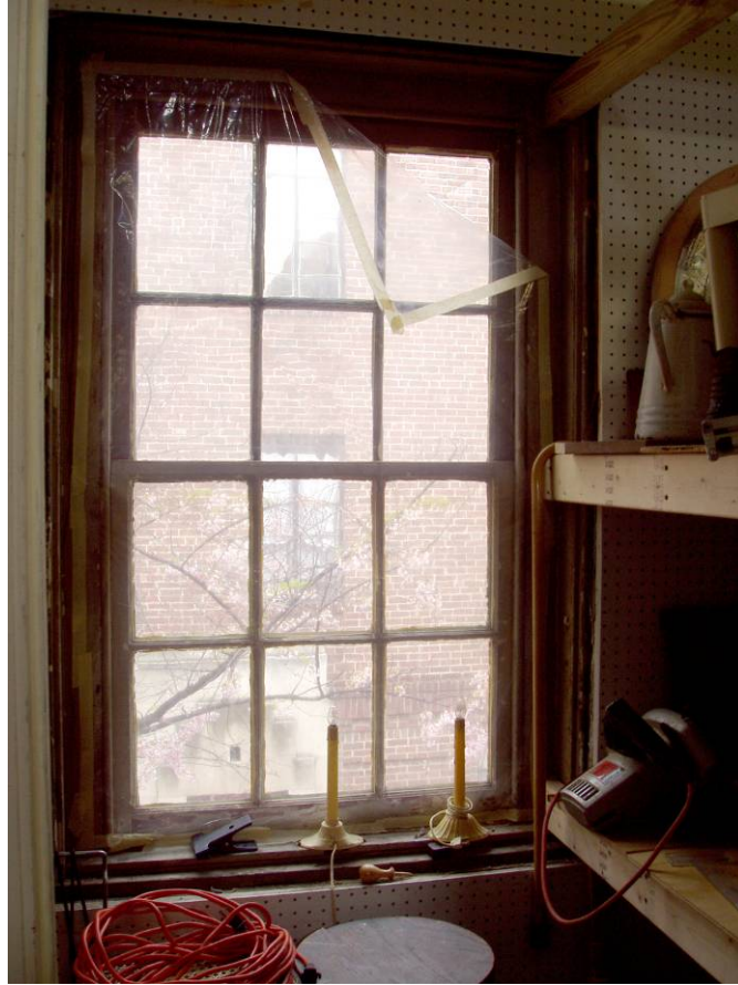
Figure B90. Second floor studio, front window inside the closet. These windows have only recently been opened, and the woodwork has not be repaired or repainted.
