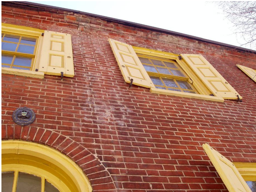
Figure B9. Exterior façade of 247 S. Camac Street, detail of the cornice and efflorescence on the brick.
