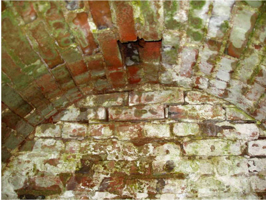
Figure B24. Rear garden retaining wall, northern vaulted storage area. Note the opening in the ceiling.
