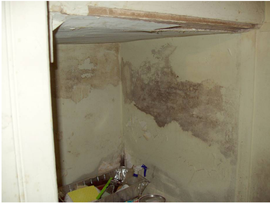
Figure B30. Basement restroom, northeast corner underneath the stairs. Note the water damage on the walls and ceiling.
