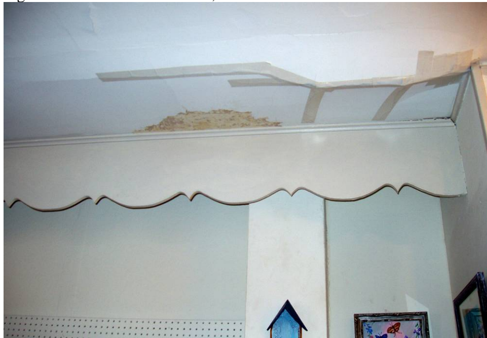
Figure B75. First floor tea room, southwest corner ceiling showing damage and fallen plaster.
