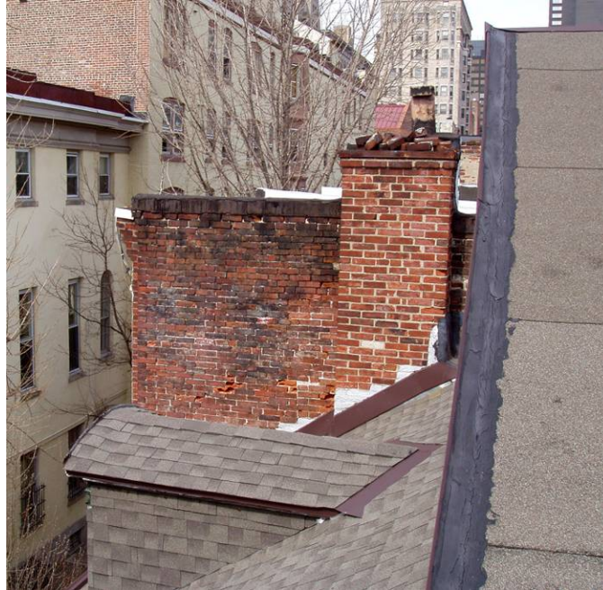
Figure B99. Roof and party wall, looking north. Note the areas on the brick wall showing mortar and brick loss.
