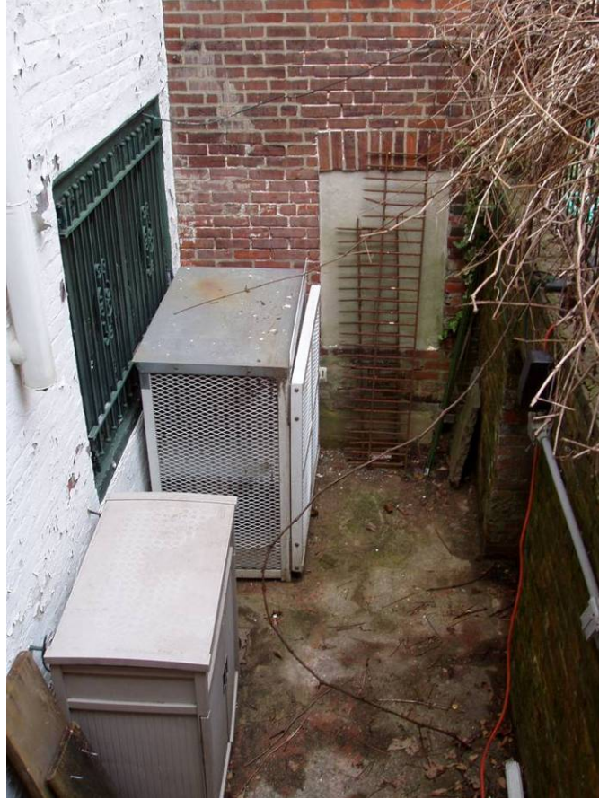
Figure B19. Rear façade, basement level passageway, looking north. Note the window to the basement restroom filled with concrete and the green biogrowth on the brick walls and concrete floor.
