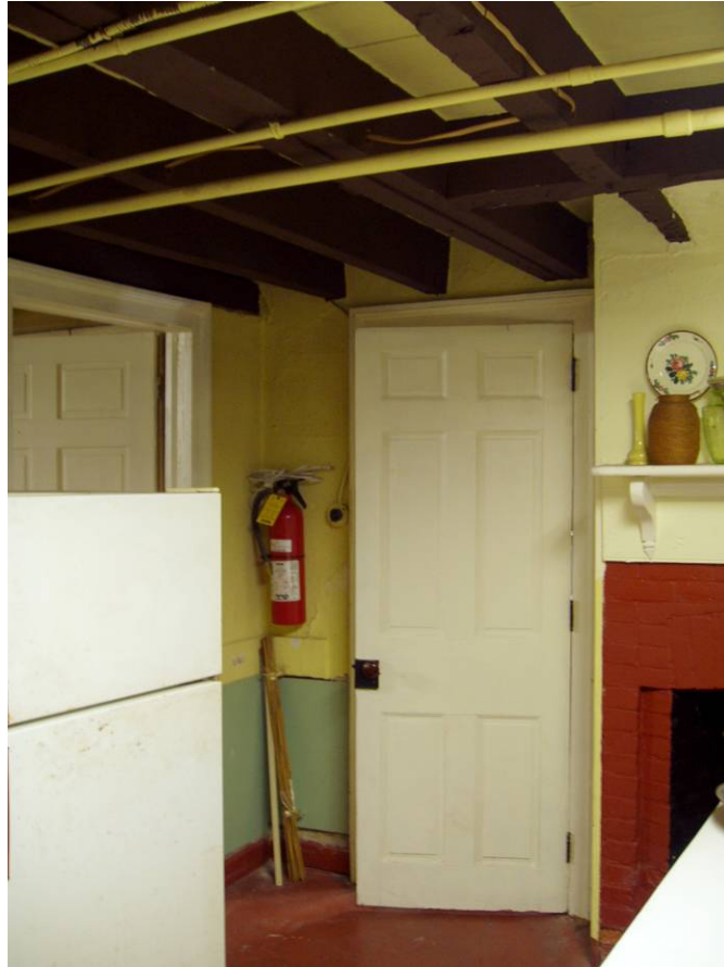
Figure B48. Basement kitchen, looking northwest. Note the water pipes and electrical lines running along and through the ceiling beams, also the green sheetrock patch along the lower portion of the wall.
