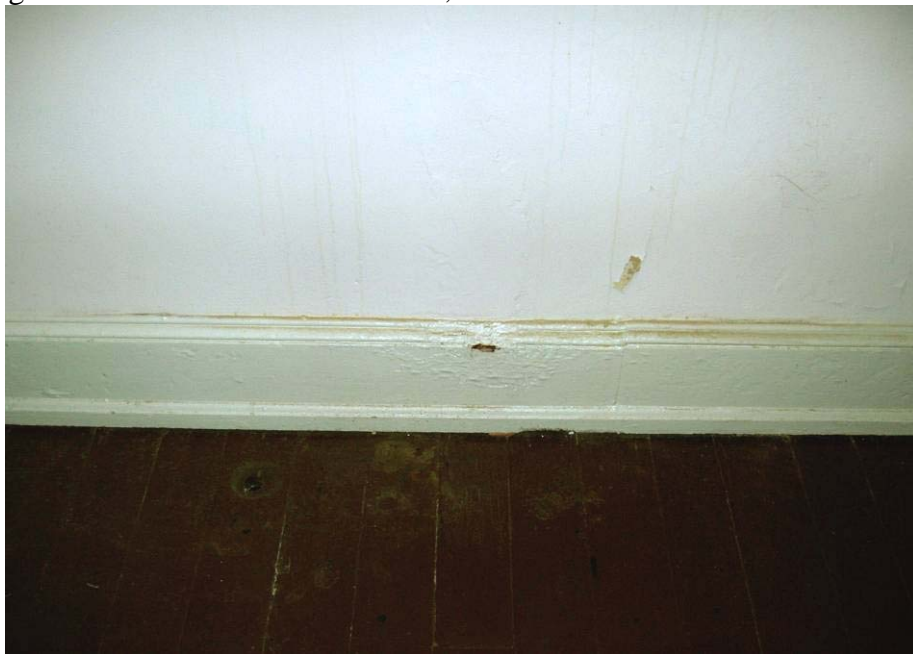
Figure B68. First floor Board Room, lower portion of the center of the west wall, showing heat damage from the original radiators.
