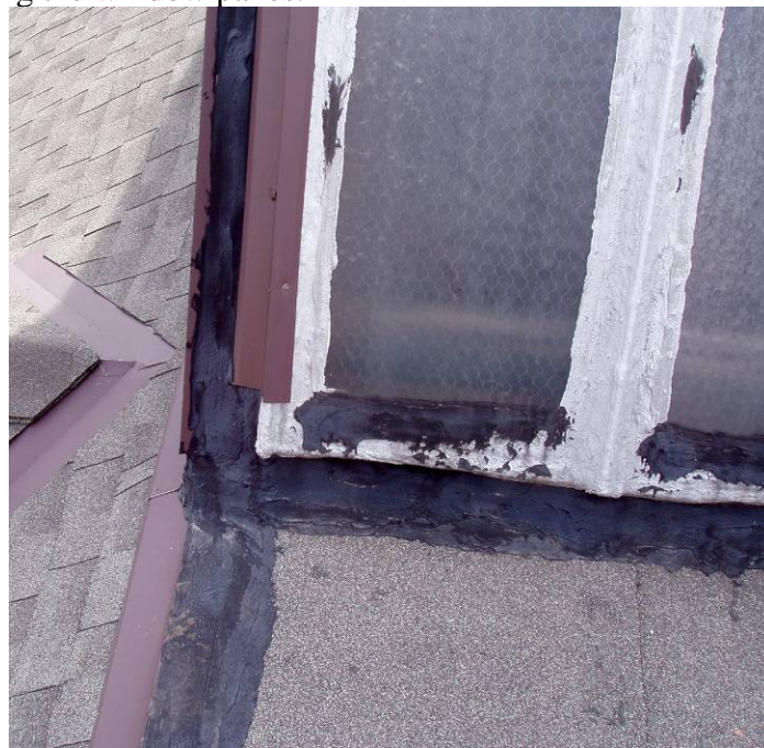
Figure B102. Skylight exterior, eastern corner. Note the buildup of tar in the attempt to fix the leak, but the flashing is incomplete.
