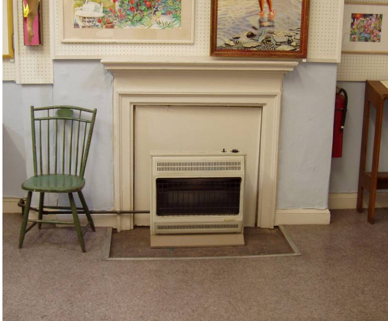
Figure B85. Second floor studio, northeast fireplace with gas-burning space heater. This unit is to be removed after the installation of the HVAC unit.
