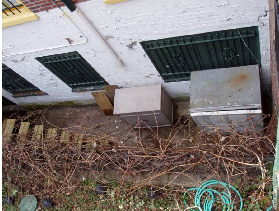
Figure B20. Rear façade, basement level passageway. Note the peeling paint and closed windows at the basement level.
