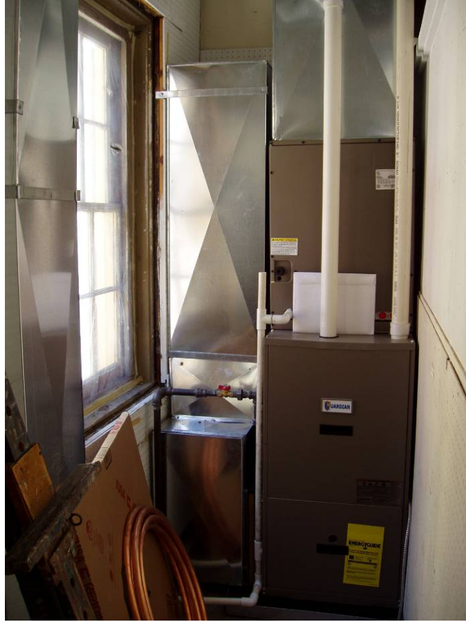
Figure B97. Second floor studio, newly installed HVAC unit in the northwest corner in the closet.
