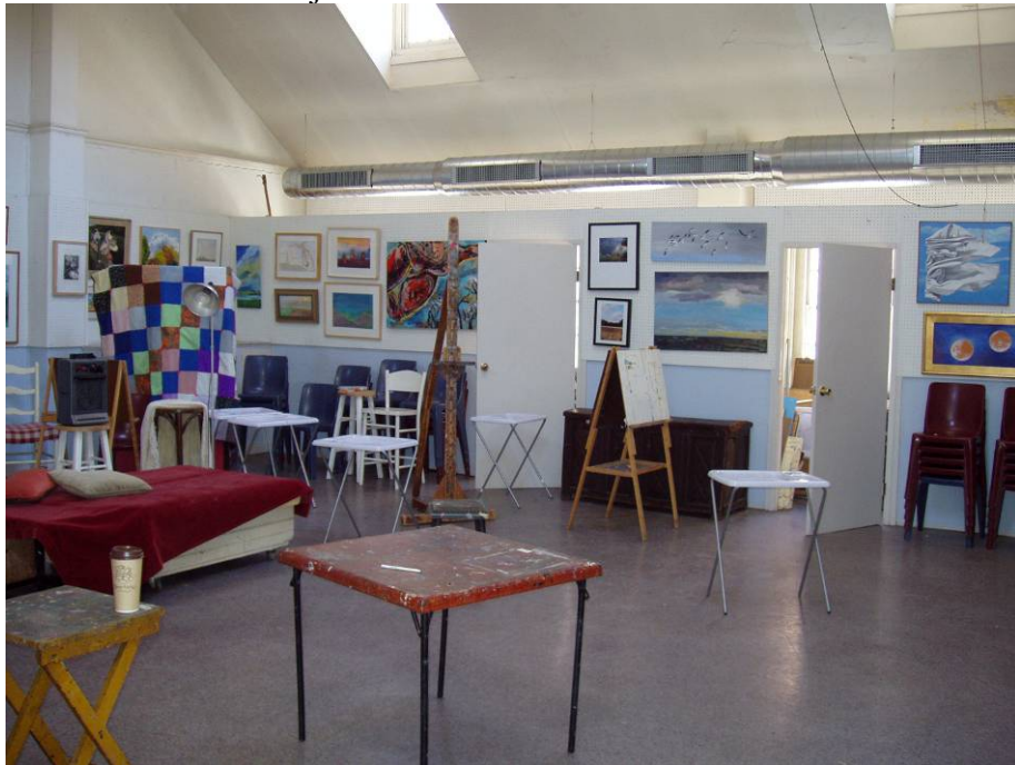
Figure B82. Second floor studio, looking southwest. Note the new aluminum duct running above the closet along the wall.
