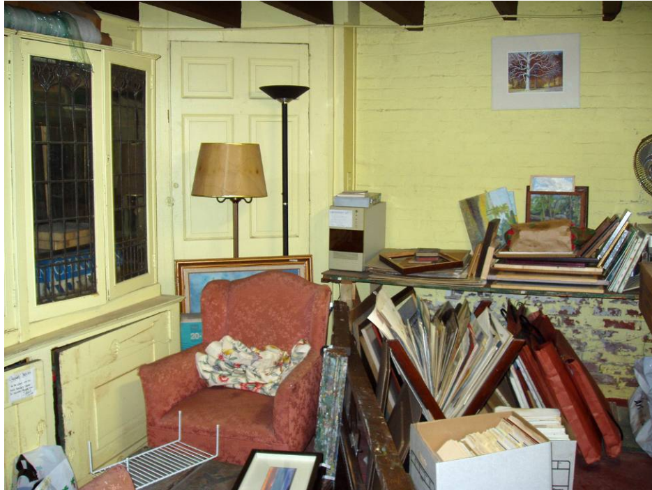
Figure B38. Basement office, former tea room, looking south. Note the water damage and peeling paint on the brick wall below the table.
