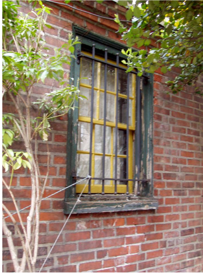
Figure B18. Rear (east-facing) window of the restroom extension. Note the paint loss and wood deterioration on the window frame.
