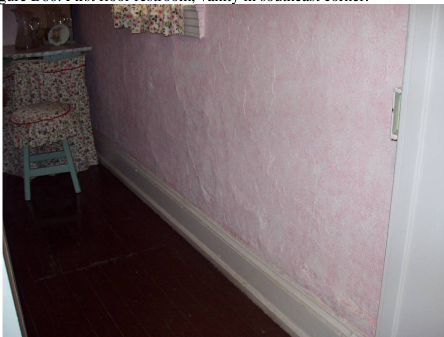
Figure B61. First floor restroom, south wall. Notice the cracks in the wall plaster.
