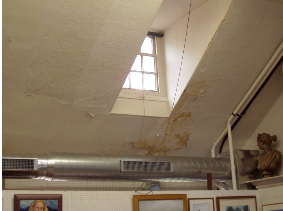
Figure B95. Second floor studio front north dormer window. Note the water damage and peeling on the plaster walls, also the piping into the HVAC unit at the right.
