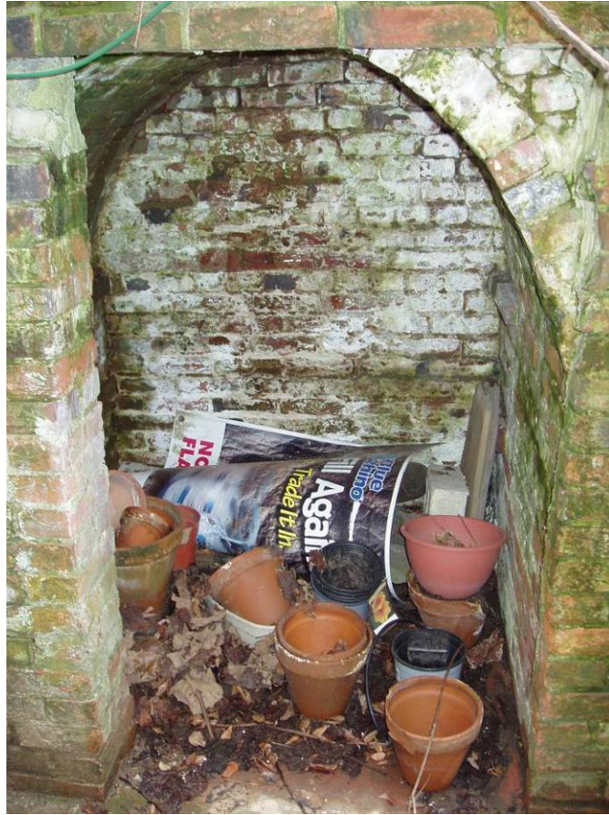
Figure B22. Rear garden retaining wall, northern vaulted storage area. Note the white staining and green biogrowth.
