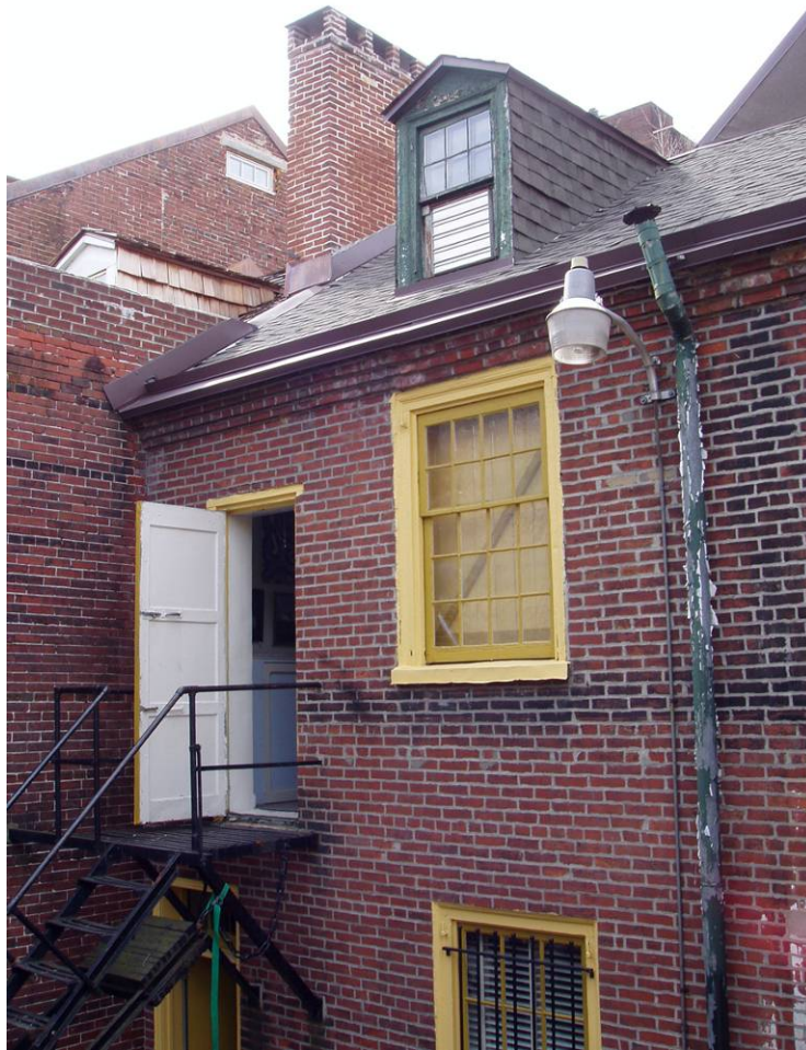
Figure B11. Rear façade, southern half. Note the poor condition of the dormer window.
