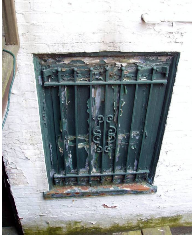
Figure B21. Rear façade, southernmost basement window. Note the peeling paint on the shutters and the green biogrowth growing at the bottom of the wall.
