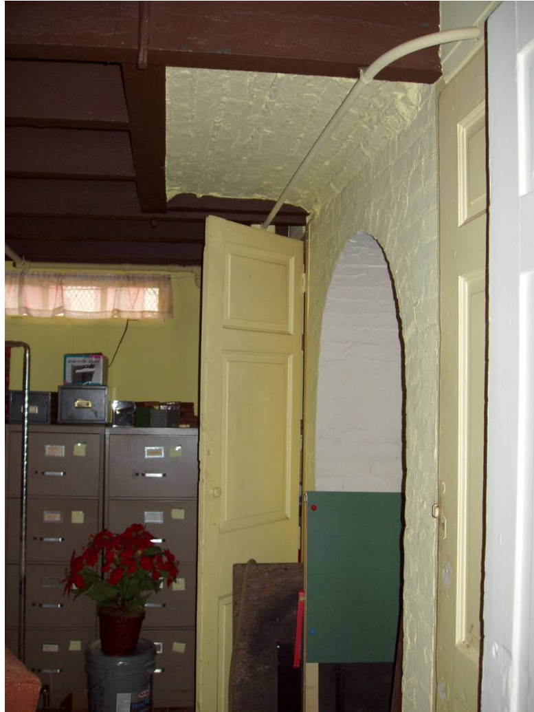
Figure B41. Basement office, former tea room, northeast corner. Note the framed brick support above the archway, indicating a support for a fireplace above. It is probable that a fireplace below this was removed for the addition of this arch.
