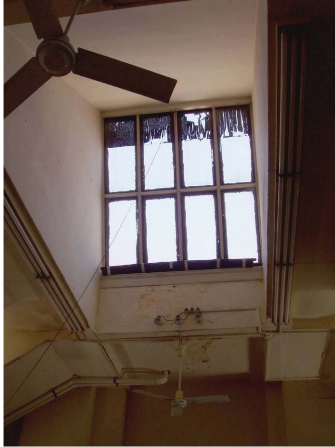
Figure B86. Second floor studio skylight. Note the blackout shade at the bottom of the window and the draw cord hanging from the top, the paint peeling from the upper portion of the window.
