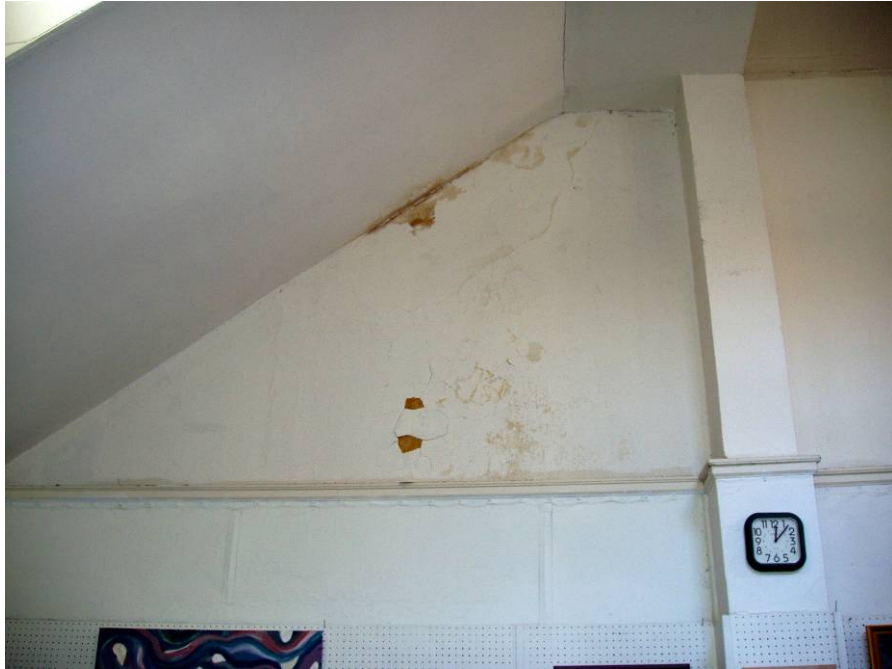
Figure B89. Second floor studio, southeast wall showing cracking and water damage.
