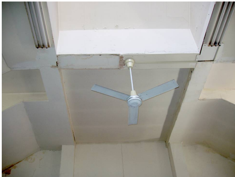
Figure B88. Second floor studio ceiling and skylight, south section. Note more water damage in the ceiling and along the top of the south wall.
