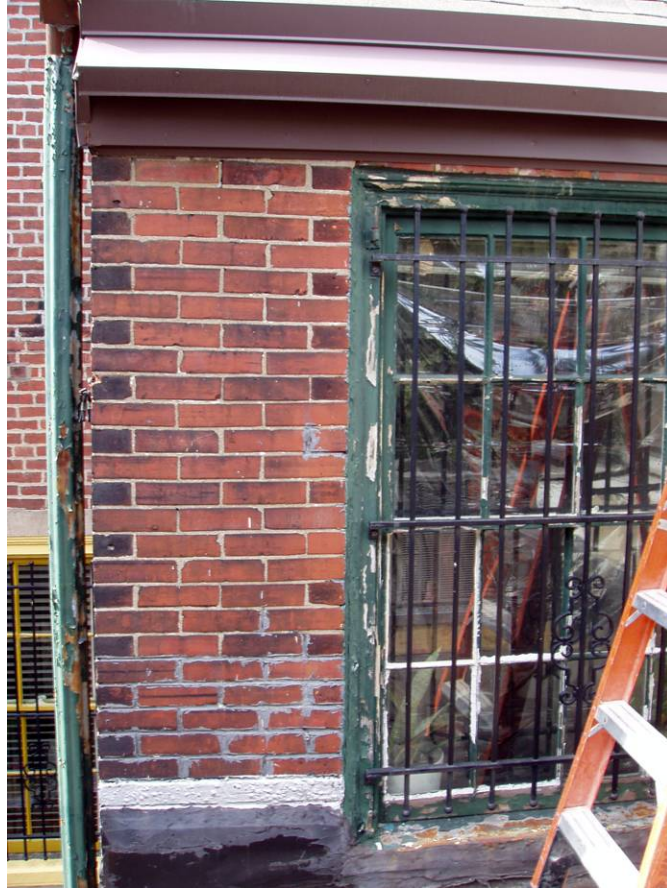
Figure B17. Rear façade of the stairwell extension, window of the landing at mid-level. Note the peeling paint and areas of decay on the wood window frame.
