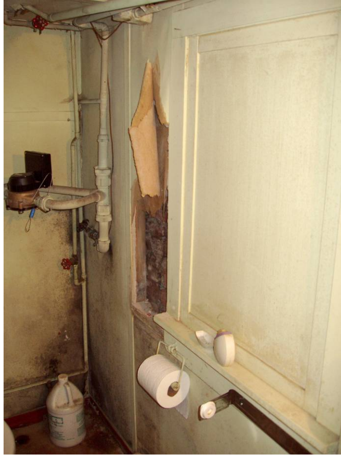
Figure B29. Basement restroom, southeast corner. Note the sever water damage on the walls.
