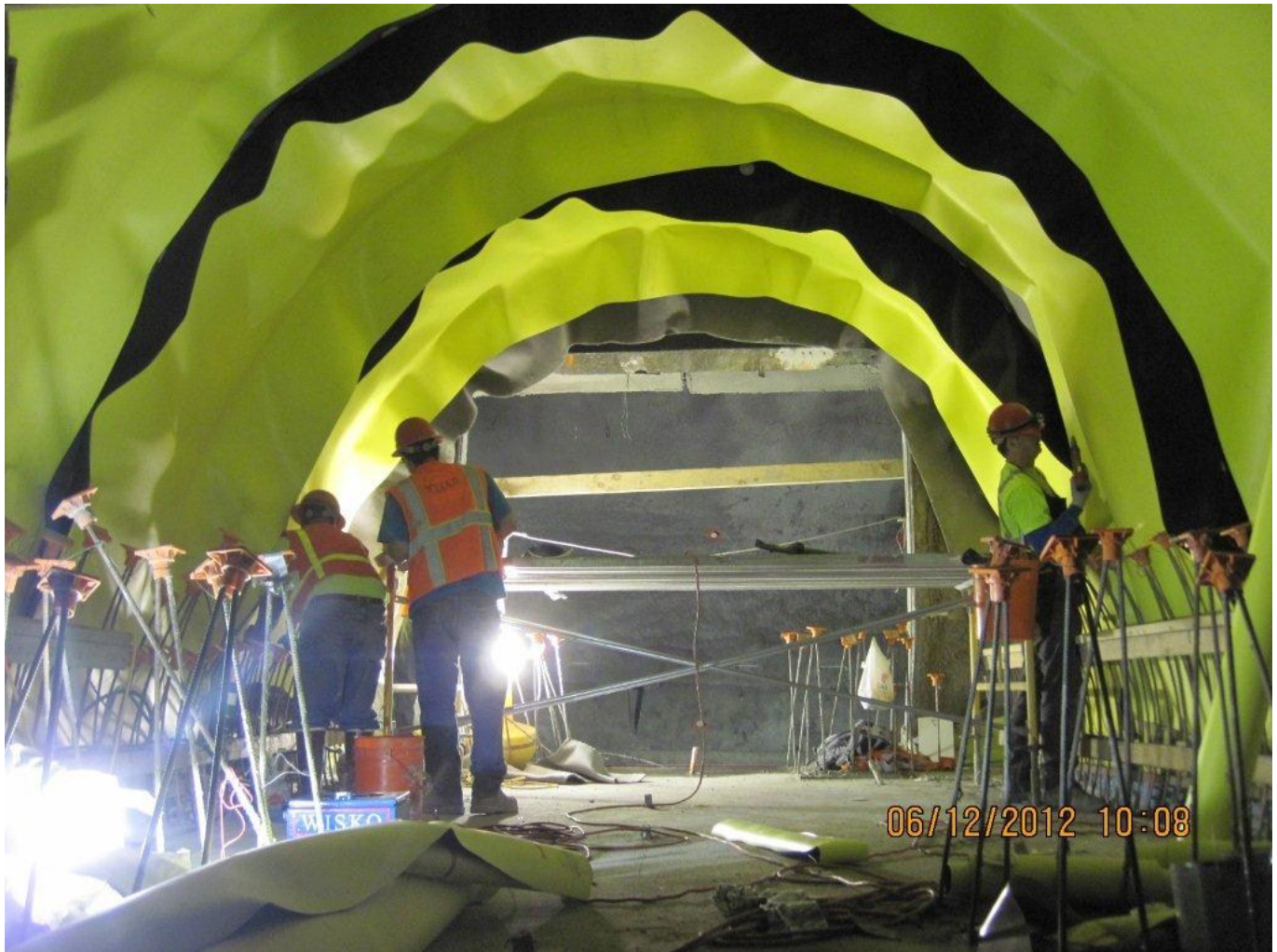
At the University of Washington Station site, arch waterproofing is installed at cross passage 19.
