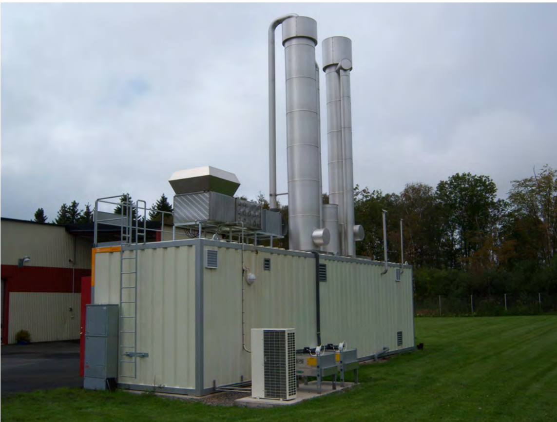
Picture 4: Biogas upgrading plant Falköping [IWES].
