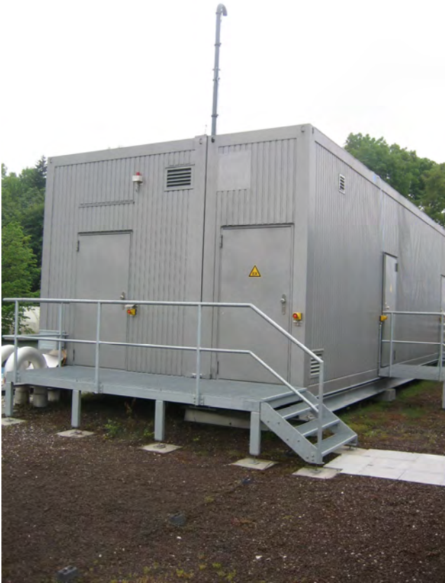
Picture 2: Biogas upgrading in Lucerne.
