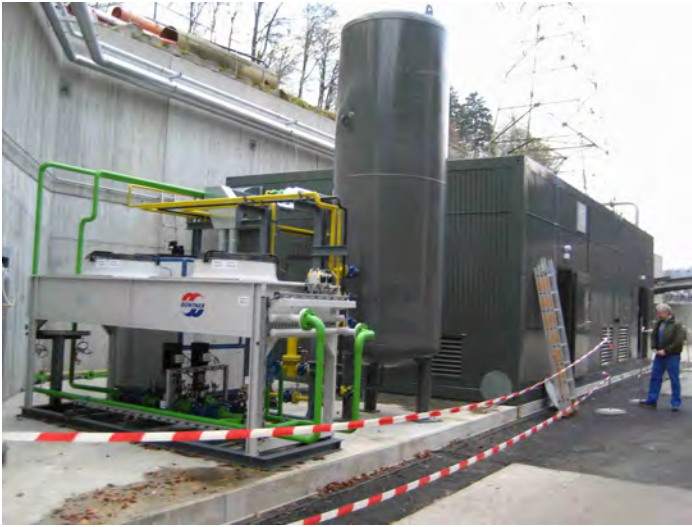
Picture 1: Biogas upgrading in Berne.
