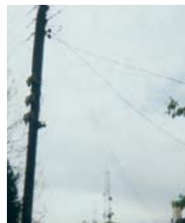
Unsightly overhead wires
