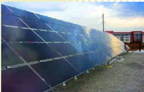
Solar Station in Krapivenskiye Dvory
