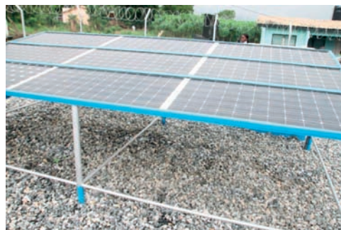
Ecobank supported Solar panel for street lights and Borehole water pump in Kojo Ashong, Ghana
