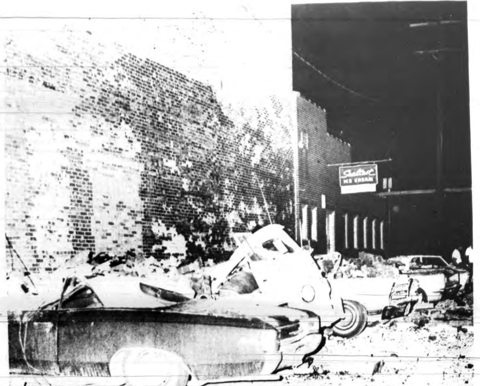
AUTOS DEMOLISHED — These cars were damaged when a wall of the Geneva Refrigerating Corp. collapsed at approximately 11:20 p.m. last night. The cars, owned by the third shift employees of the American Can Co., were
