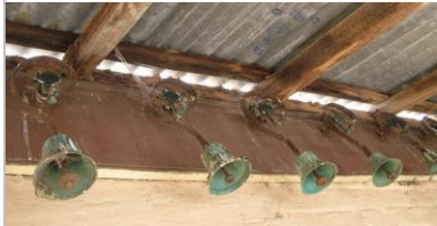
Servants Bells at Woolmers Cottage (before restoration). © DEPHA
