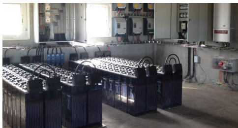
AC coupled PV/Diesel/Batteries Hybrid system implemented at Isona (Lerida), Spain by Granjes Pereto
