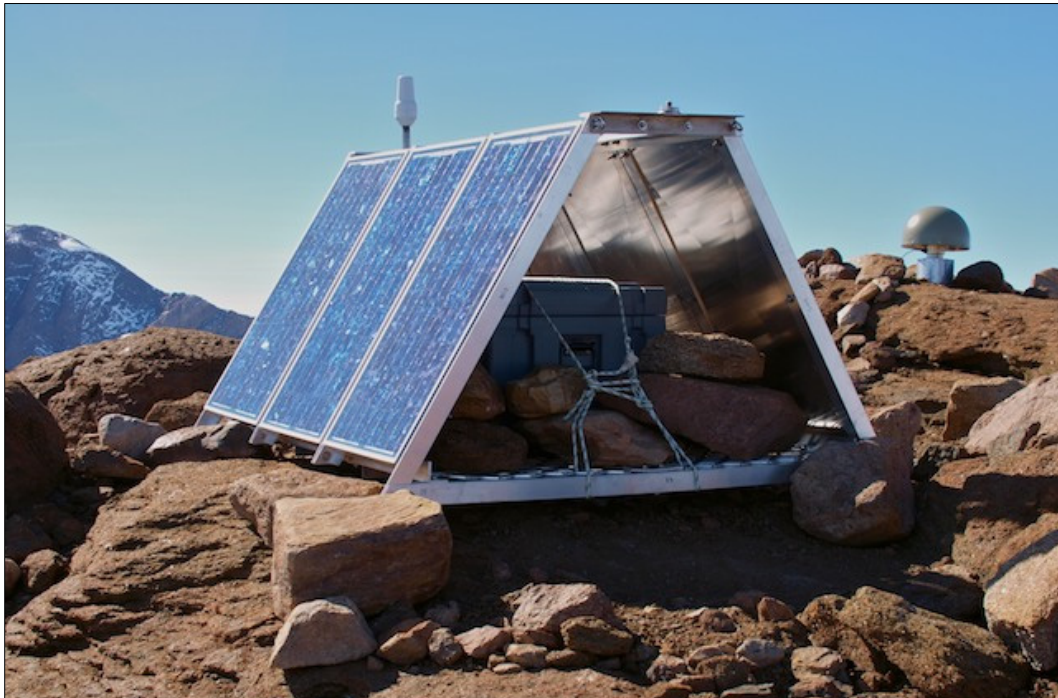
Figure 5.2: Solar panel frame structure, as installed at the Grove Mountains (December 2009).
