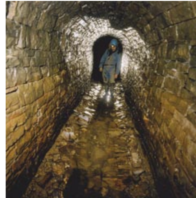
This fine arched level at the Ecton Mines near Warslow leads to the heart of one of the most exciting survivals underground, where there are engine chambers and many other features. In the late 18th century it was one of the richest mines in Britain (© Paul Deakin).
