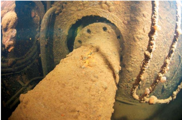
Shafting leading to dislocated Flange F inside Thrust Block enclosure
