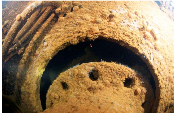
Flange F can be seen here completely 'dislocated' from the Thrust Block.
