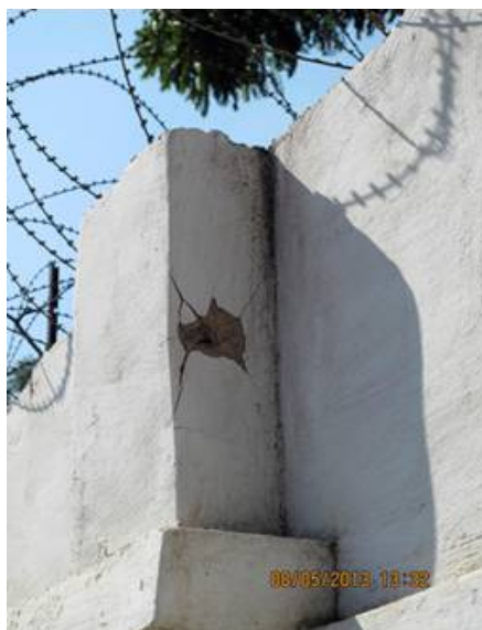
Bullet hole in the wall of the MONUSCO Headquarters, shot by FARDC on 23 March 2013.
