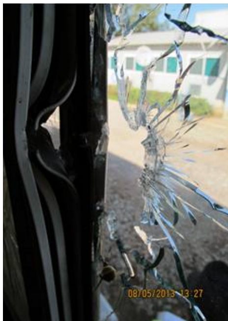
Window in MONUSCO's Security Office smashed by a bullet fired through the main gate of the MONUSCO Headquarters in Lubumbashi on 23 March 2013.
