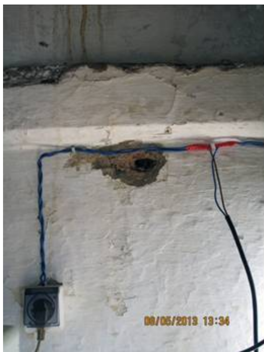
Bullet hole in the front gate of the MONUSCO Headquarters in Lubumbashi, shot by a FARDC soldier on 23 March 2013.
