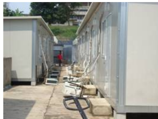
Air conditioners ripped out of the walls of MONUSCO housing for security personnel by protesters who breached the west fence of the ONATRA base on 20 November. (UN staff)
