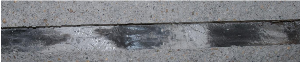
Figure 31 – The face of the concrete casing is clearly marked by the buckled steel core
