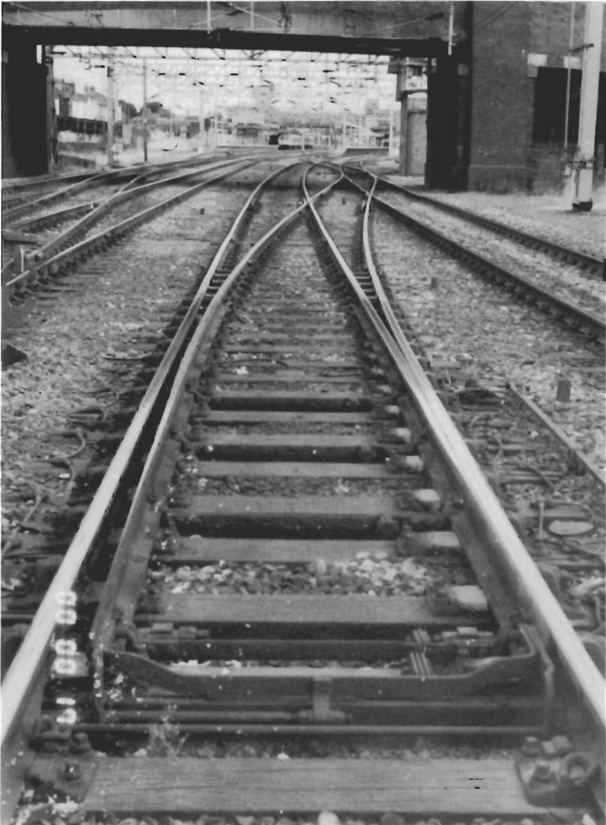
Figure 4 View from Up Slow line of Bridge No 86, Stafford 5 Signal box and Stafford Station
