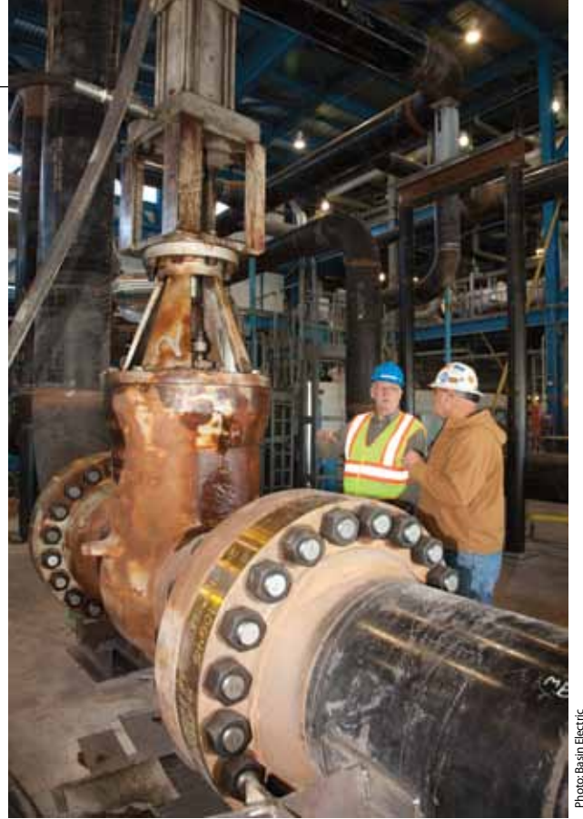
Photo: Basin Electric
