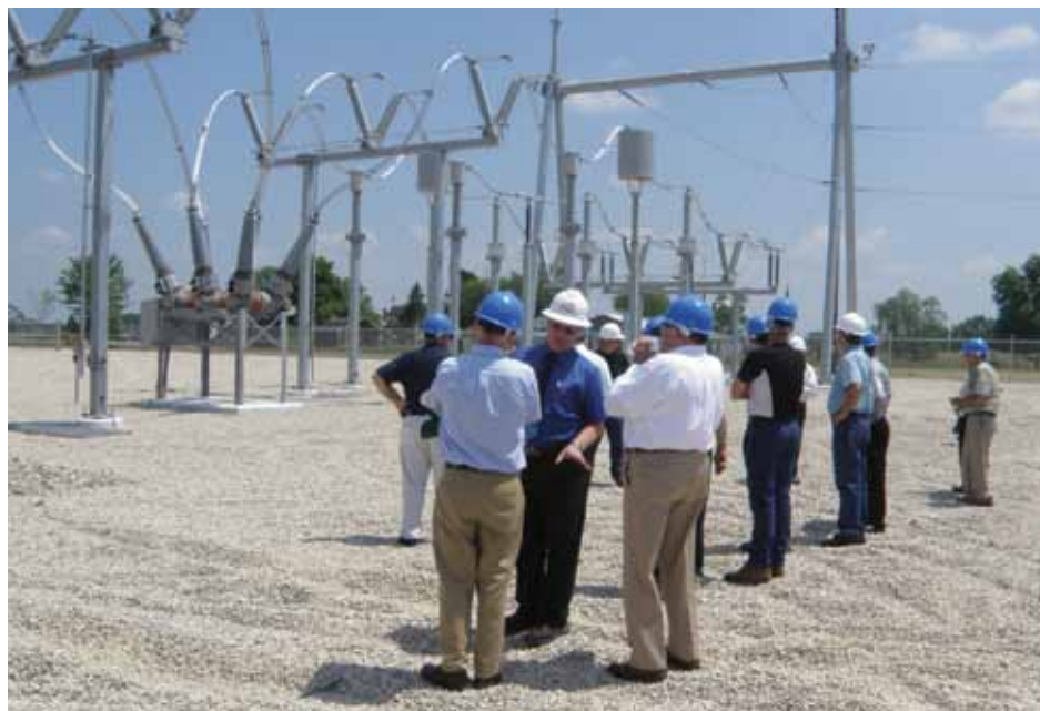
HomeWorks’ board of directors toured Wolverine’s Clinton Interconnection, at Clinton Trail (M-50) and Mulliken Highway, soon after its completion in May 2010. The project upgraded transmission service to Eaton and Ionia counties.
