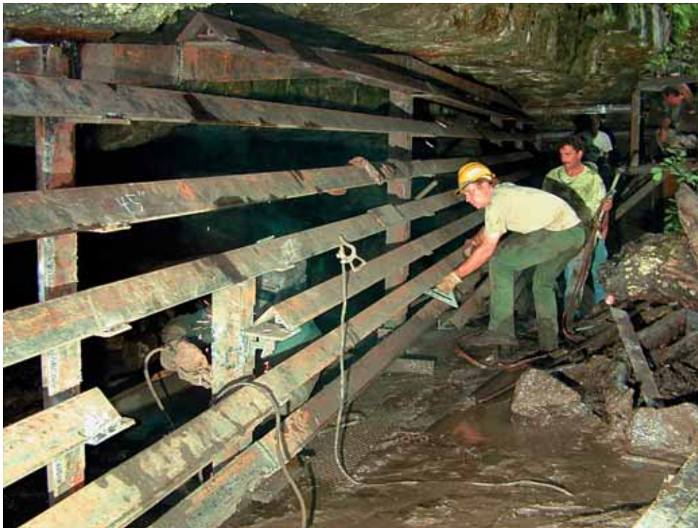
FIGURE 4 A cave-gating class builds a bat-friendly cave gate at McDowell Cave in Missouri. Note the T-bar stiffeners inside the end of the top horizontal bar which provide greater strength and an airfoil design for lower wind resistance. Proper spacing of the bars is essential.
