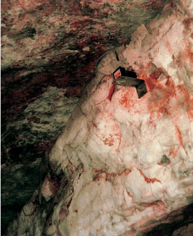
FIGURE 2 Sometimes joints in a cave indicate the possibility of future rock falls. In order to ensure the safest conditions in a show cave, it is necessary to detect well in advance any minor movement. A detector that monitors possible displacement of a limestone layer can be seen in this photograph of Kartchner Caverns in Arizona. (Photograph courtesy of Arrigo A. Cigna.)
