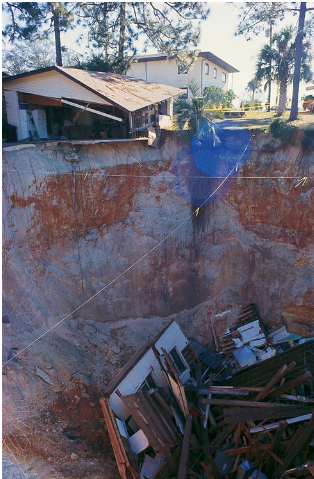
FIGURE 3 The remnants of a home engulfed as a large cover-collapse sinkhole developed over several hours, Keystone Heights, Florida (east of Gainesville). The occupants were able to evacuate safely, although their Christmas tree and presents were lost. The surficial sediment is clayey sand, which spans the upward eroding subsurface void allowing it to grow to a significant size before it collapsed. The limestone at this location is approximately 100 feet below the land surface. (Photograph courtesy of Barry F. Beck.)
