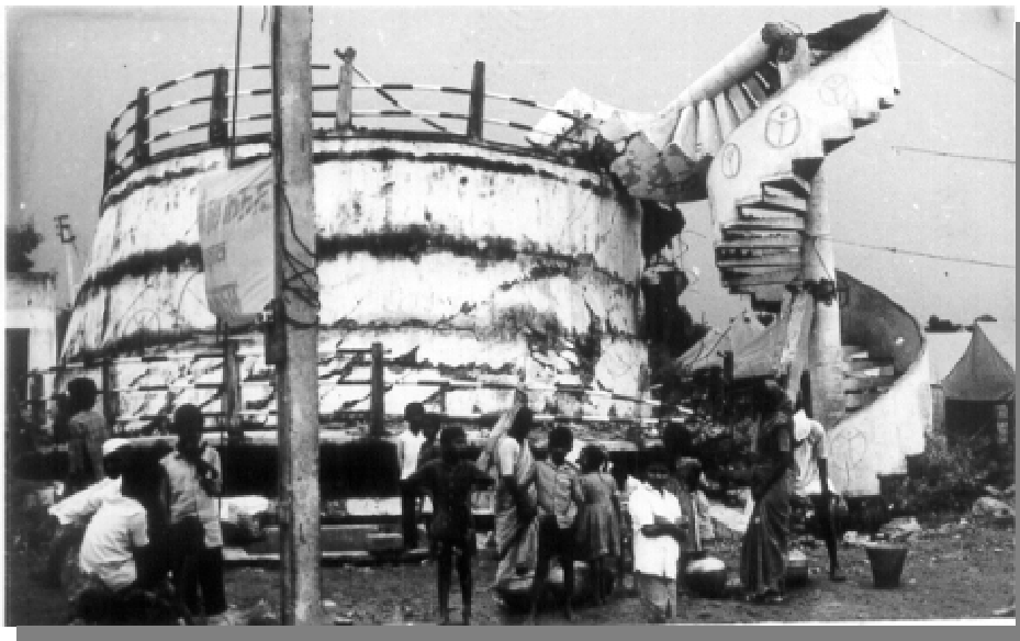
Figure 6: While most elevated water tanks performed well, this tank of Kautha collapsed straight down into its crumpled supports. Circumferential displacement of about 0.5m suggests that rotational vibration led to its collapse.
