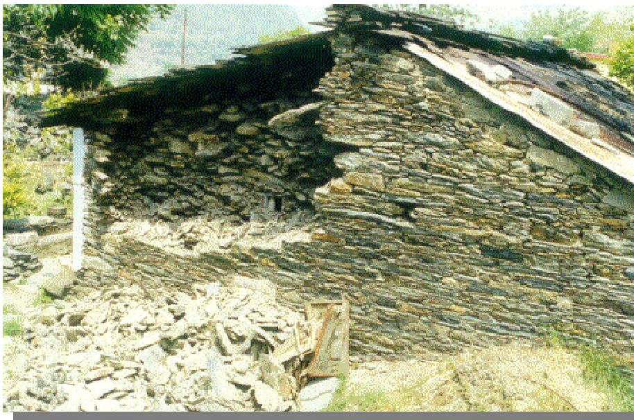
Figure 7: Collapse of one of the wythes in a traditional house in slate wafer masonry.
