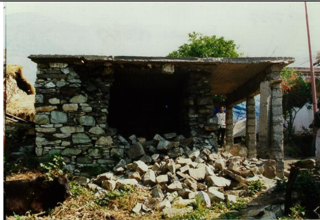
P1. Partial collapse in a random rubble stone masonry building. Note that the front portion has RC beam supported on concrete block columns, and that the roof consists of an RC slab.
