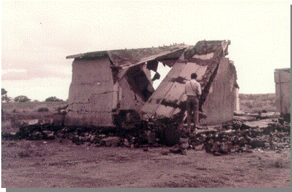
Figure 5: A brick masonry school building in Rajegaon collapsed. The roof of precast panels lacked adequate connections
