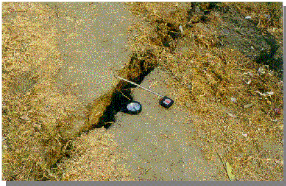
Figure 5: Ground fissure at Telecom Hill near Gopeshwar
