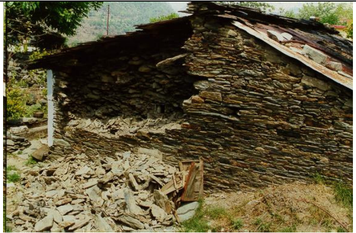
P2. Collapse of one of the wythes in a traditional house in slate wafer masonry
