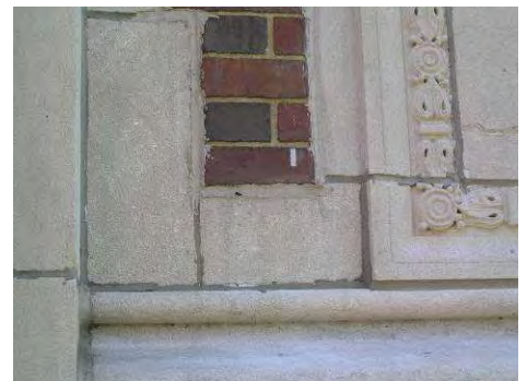
Figure 106: The pointing mortar used in this stone repair at D. M Smith does not appear to match the historic mortar.
