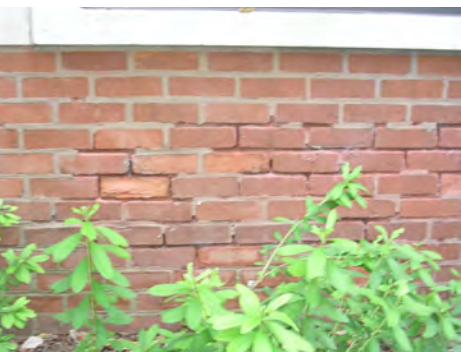
Figure 105: Image of significant mortar deterioration and brick spalling along the base of a historic building.
