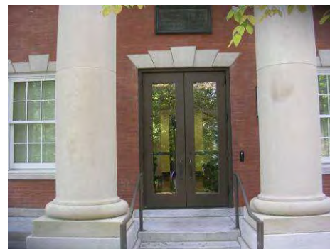
Figure 102: The installation of modern bronze doors has altered the character of this historic entryway.
