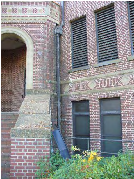
Figure 104: Biological growth and mortar deterioration associated with the location of a downspout on the O'Keefe Main Building.
