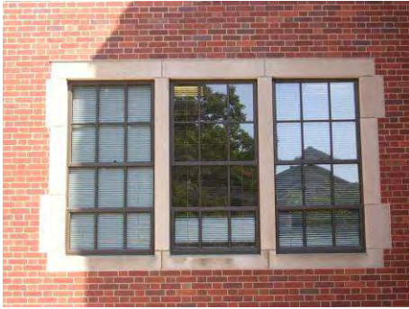
Figure 103: The character of the original multi-pane windows was replicated in the replacement units installed during the recent rehabilitation of the Old Civil Engineering Building.
