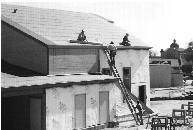
Construction on the new CSC, early 1993, with Hays County Court House in the background (CSC album)
