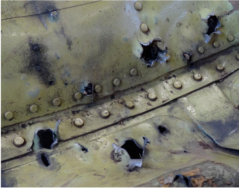
Figure 8: Plate material bent inwards. Looking at the inside of the structure
