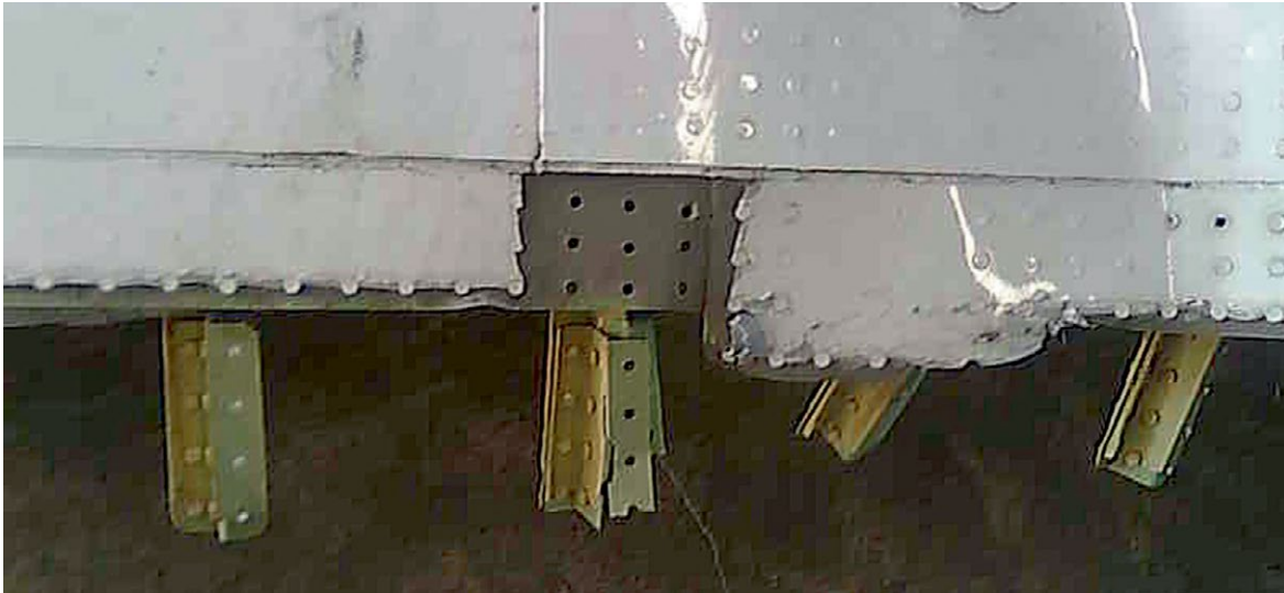
Figure 19: Pure shear failure, fracture in circumferential joint. (Source: Dutch Safety Board)
