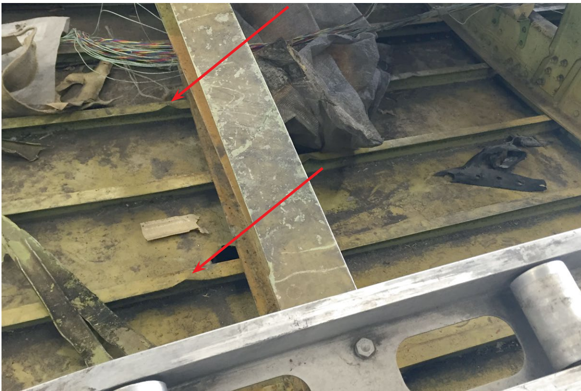
Figure 22: Illustration of stringer buckling, see red arrows, indicating compression. (Source: Dutch Safety Board)
