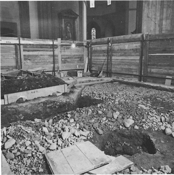
25 Octagonal base in fourth side aisle bay (zone B in Fig. 12) (photo: Soprintendenza ai Monumenti)
