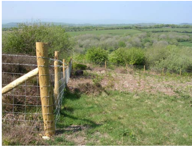
New fences and scrub clearance at one of the Mynydd Mawr Agreement sites
