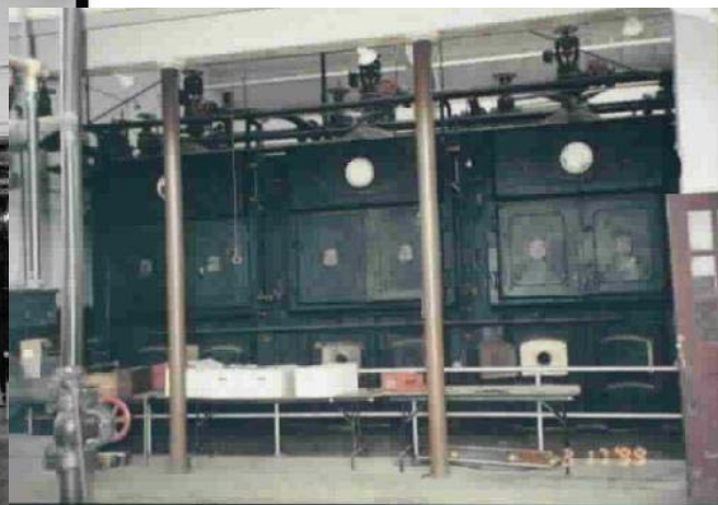
Front of three water tube boilers
