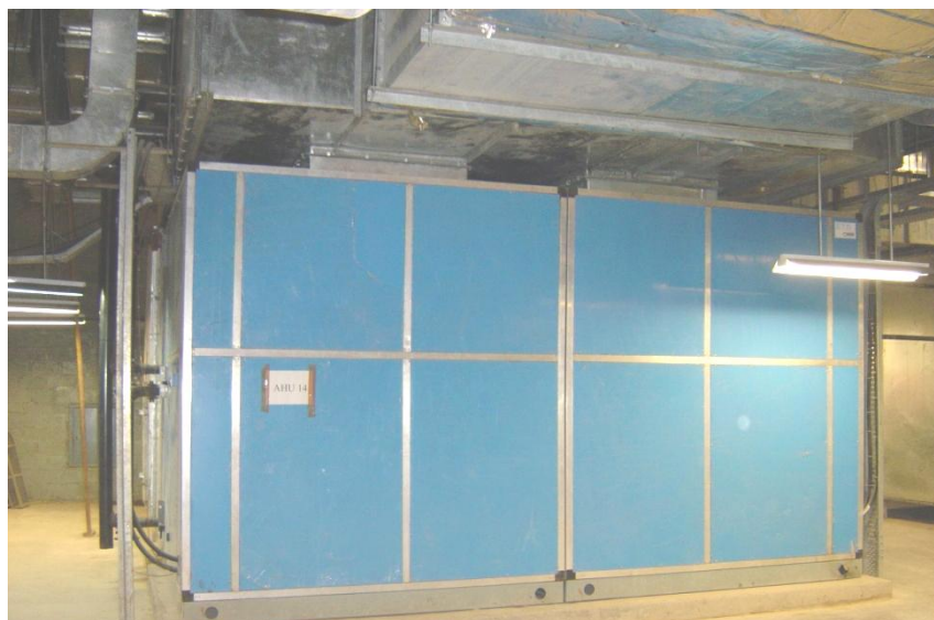
Air Handling Unit
