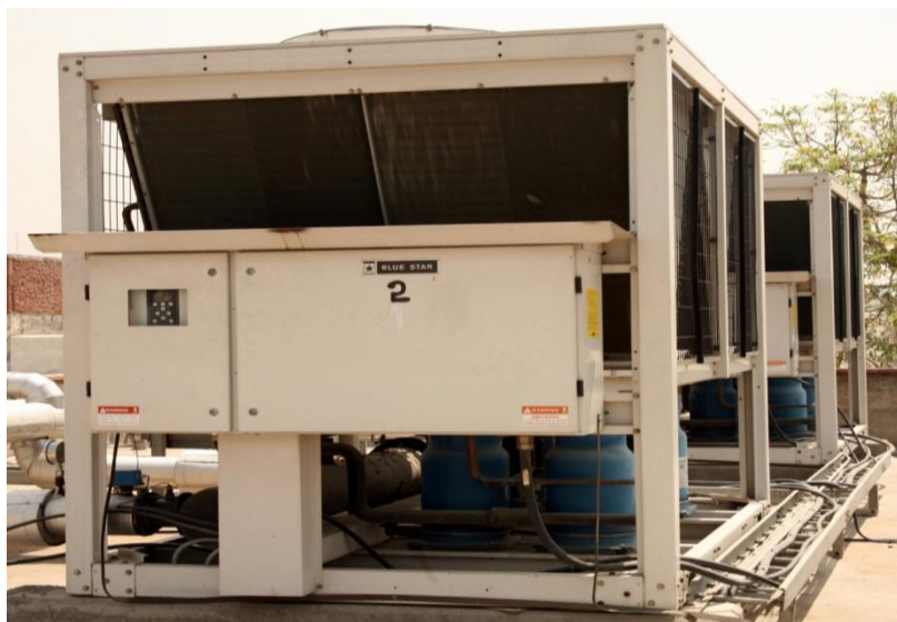
Air Cooled Chiller
