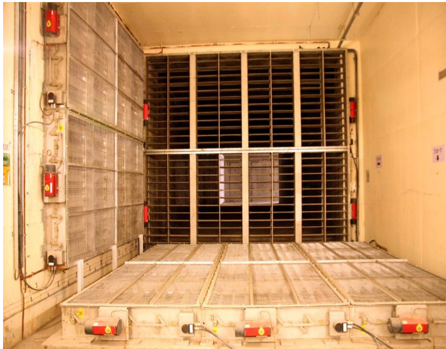
Tunnel Ventilation Dampers
