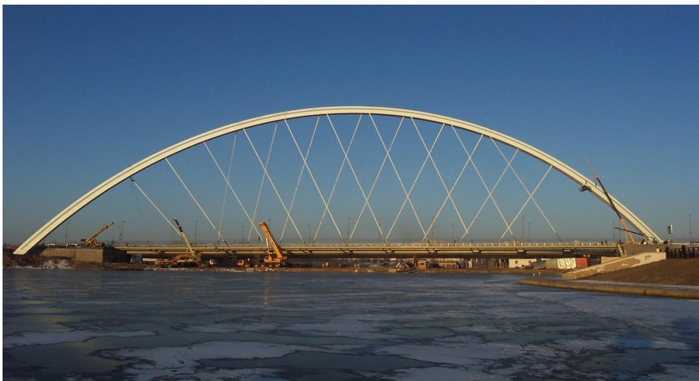
▲ Construction of a soil bund in the river enabled the deck to be built on temporary supports.
