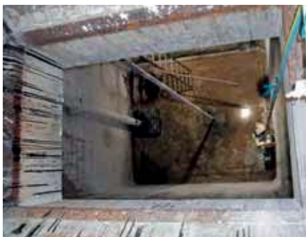
FED vault 1A at Bradwell
