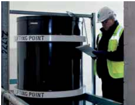
Bulk resin retrieval from resin vault two
