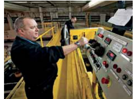
Operator moves fuel skips in the ponds
