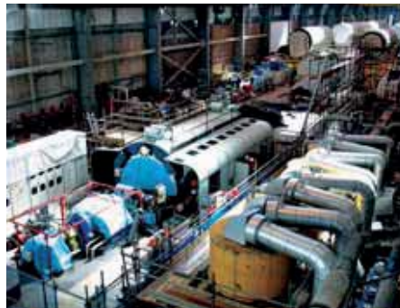
Wylfa turbine hall
