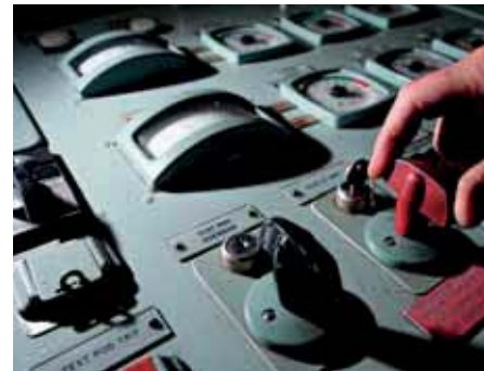
Power station control room
