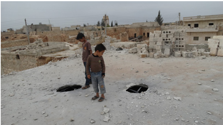
Damage caused to a home by missiles loaded with cluster munitions. Source: Civil Defense in Hayyan
