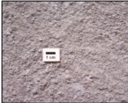
Figure 3. Indiana Limestone (also known as Salem Limestone) on the exterior of the Bank of America building.
